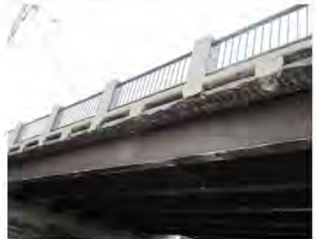
Most significant deterioration
