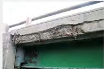
Deck Fascia Deterioration
