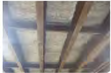
Deterioration in Bridge deck 2015
