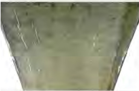
Arch Ring Map Cracking
