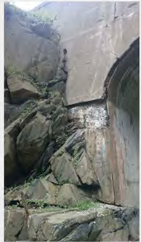
Poor Condition of the Arch Wall
