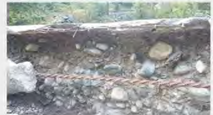
Deteriorated Bridge Railing
