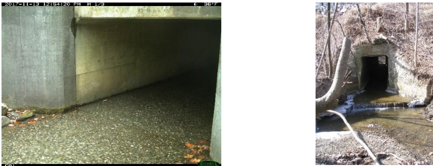
Figure 27. Examples of old box culverts with “sheetflow concrete” movement surface. Site 30-22 (West Townshend) and 15-76 (Cambridge, Marangelo and Farrelll 2016).
