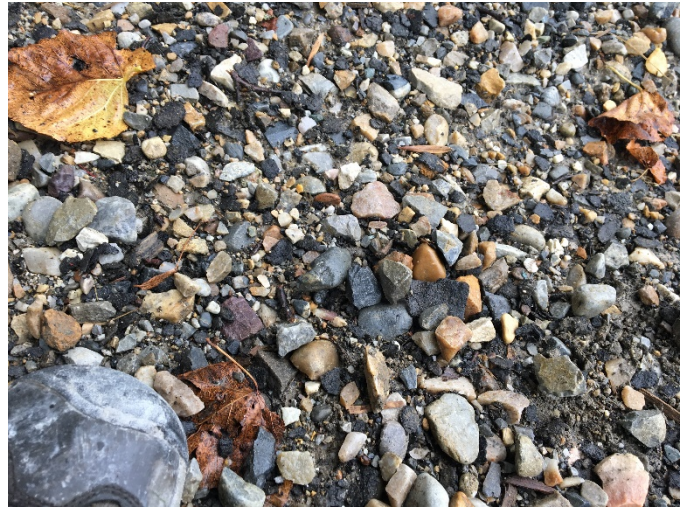
Loose Shoulder Material
