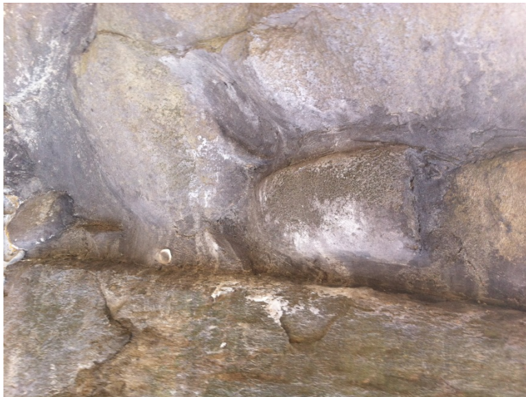
Figure 17: Up-close view of white powdery residue on mortar (2017)
