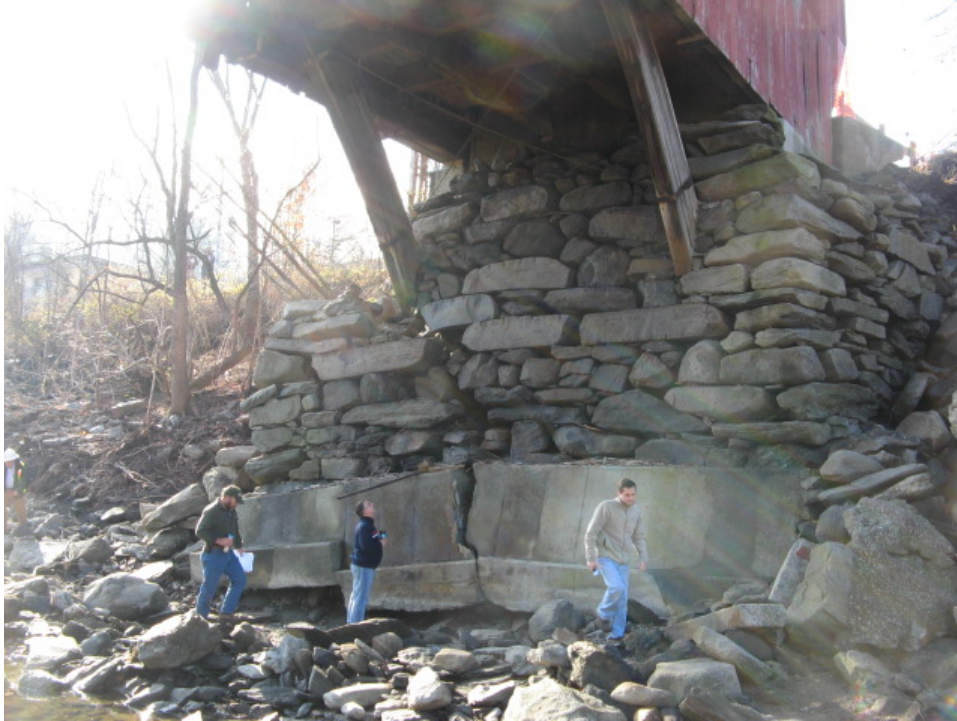
Figure 9: Western abutment partially collapsed
