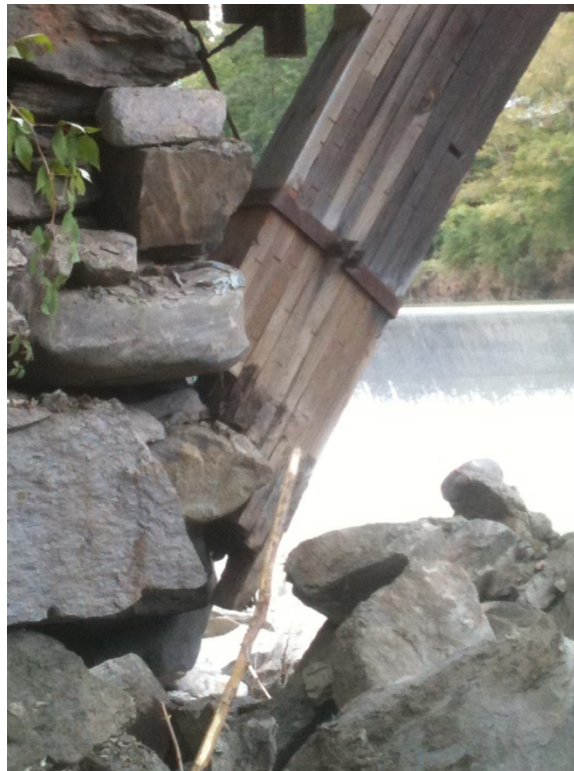
Figure 11: Downstream western arch dislodged from abutment
