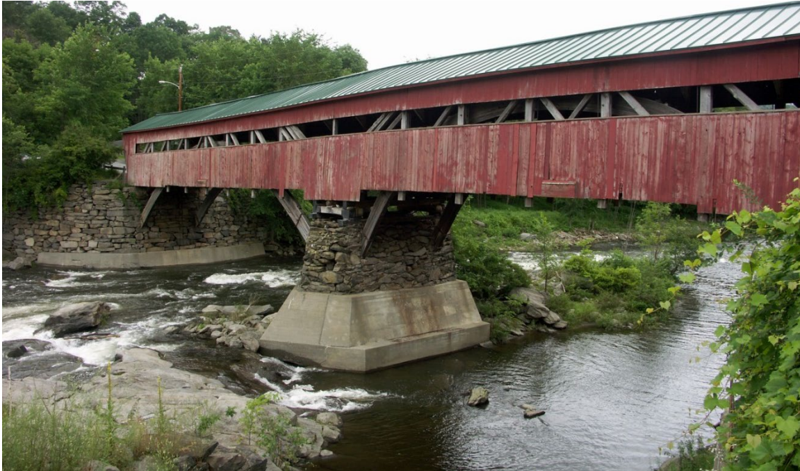
Figure 2: The Taftsville Covered Bridge in 2006 showing the Pier and Abutment that were preserved
