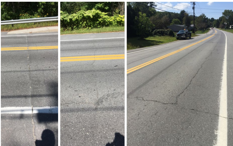
Figure 6: Cracking at western approach of Bridge 8
