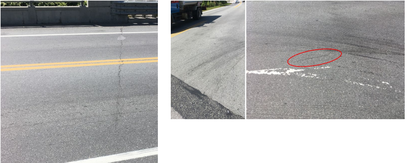
Figure 9: Cracking at the western approach of Bridge 9
