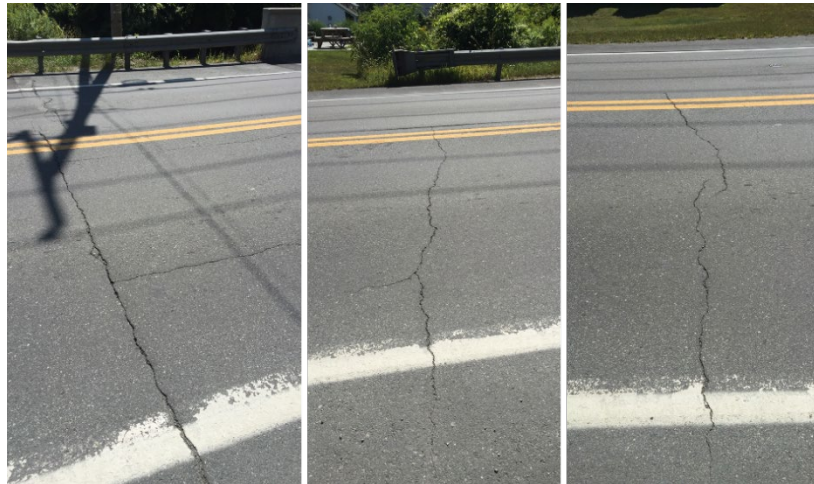
Figure 5: Cracking at eastern approach of Bridge 8
