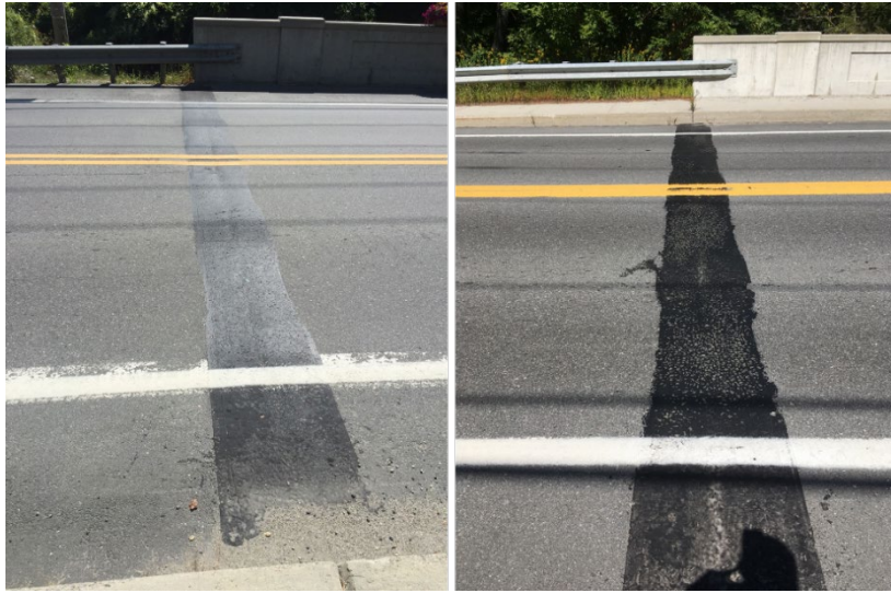
Figure 4: Bridge 8 joints, east and west ends respectively, appearing to be in good condition
