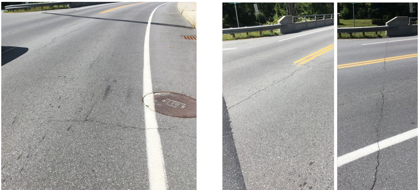
Figure 8: Cracking at eastern approach of Bridge 9
