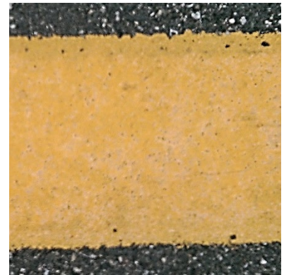
Surface Epoxy Utah, 36 months, 29-0+00
