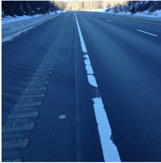
Figure 23: TS 25 Damage Overview
