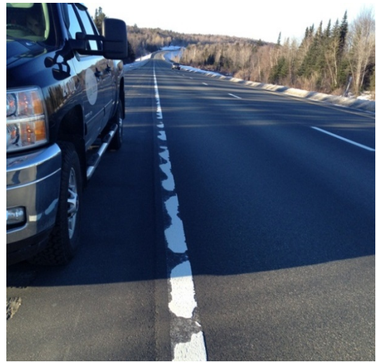
Figure 26: TS 28 Damage Overview
