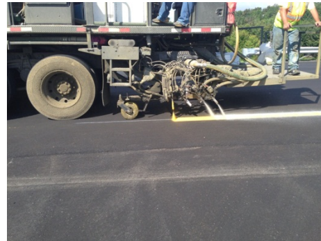
Figure 12: Yellow Epoxy binder and optic package being applied through two chutes for a double drop.
