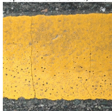
Recess Thermoplastic Wet Reflective, 8 months, 23-0+00
