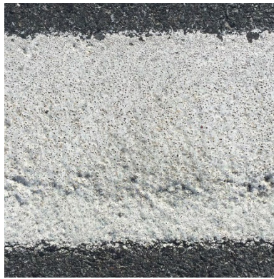
Surface Polyurea Wet Reflective, 15 months, 15-0+00
