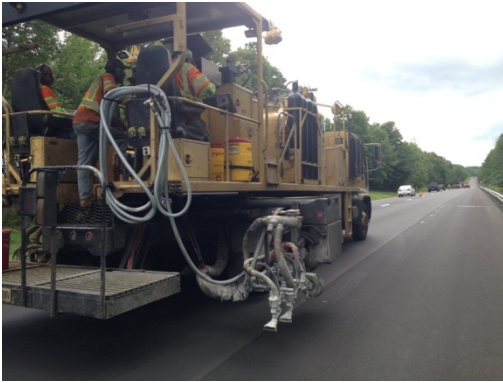
Figure 9: Polyurea application truck, featuring two chutes for application of a double drop of optics.
