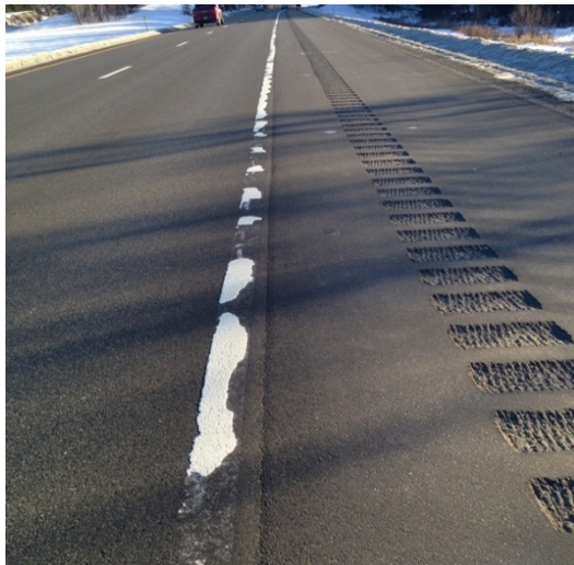
Figure 25: TS 28 Damage Overview
