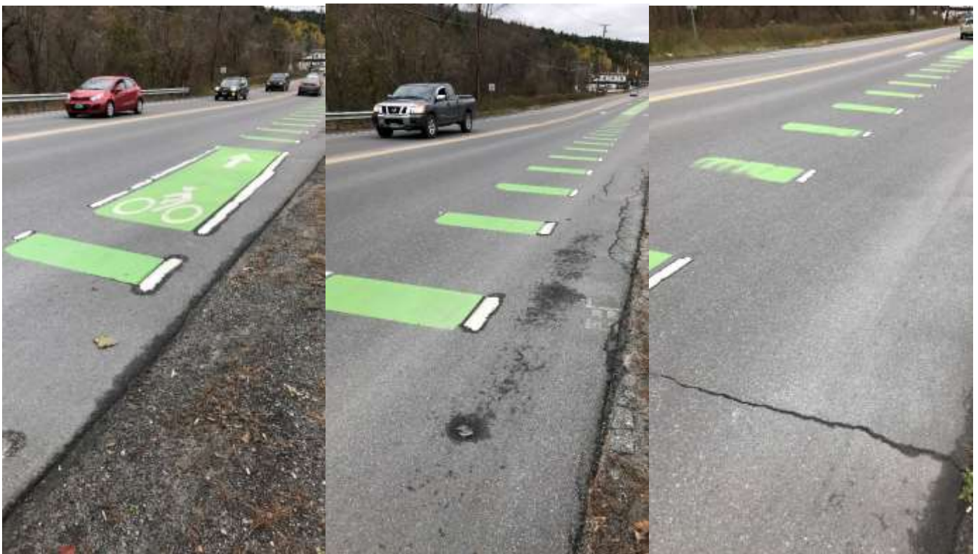
Figure 14: PreMark Condition Location 1
