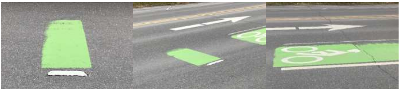
Figure 12: Location 1 PreMark in Fair Condition
