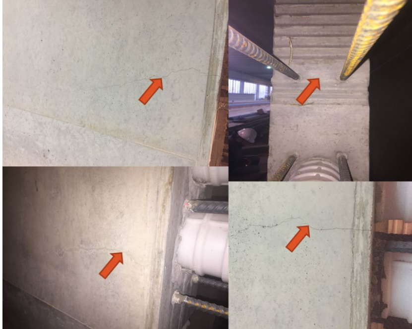
Figure 1.3: Recorded end zone cracking of bulb tee
