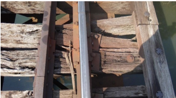
Bridge being replaced on VTR as part of 2018 BUILD Grant. Source: VRS
