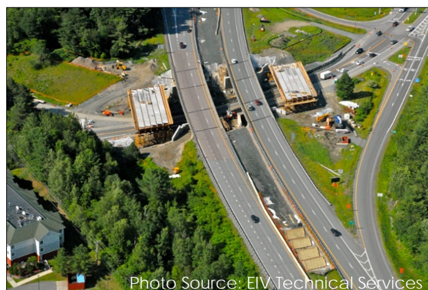
Photo Source: EIV Technical Services Figure 5: Preparations for the I-91 Bridge Slide in Hartford, VT, a unique project that featured “slide-in” bridge construction to limit downtime. This type of project makes an excellent TAC field trip.
