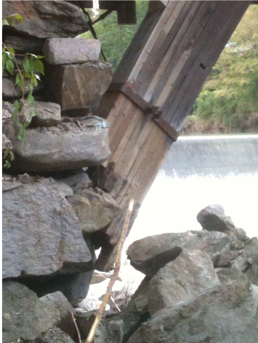
Figure 10 Downstream westerly arch dislodged from abutment (VTrans 2011)
