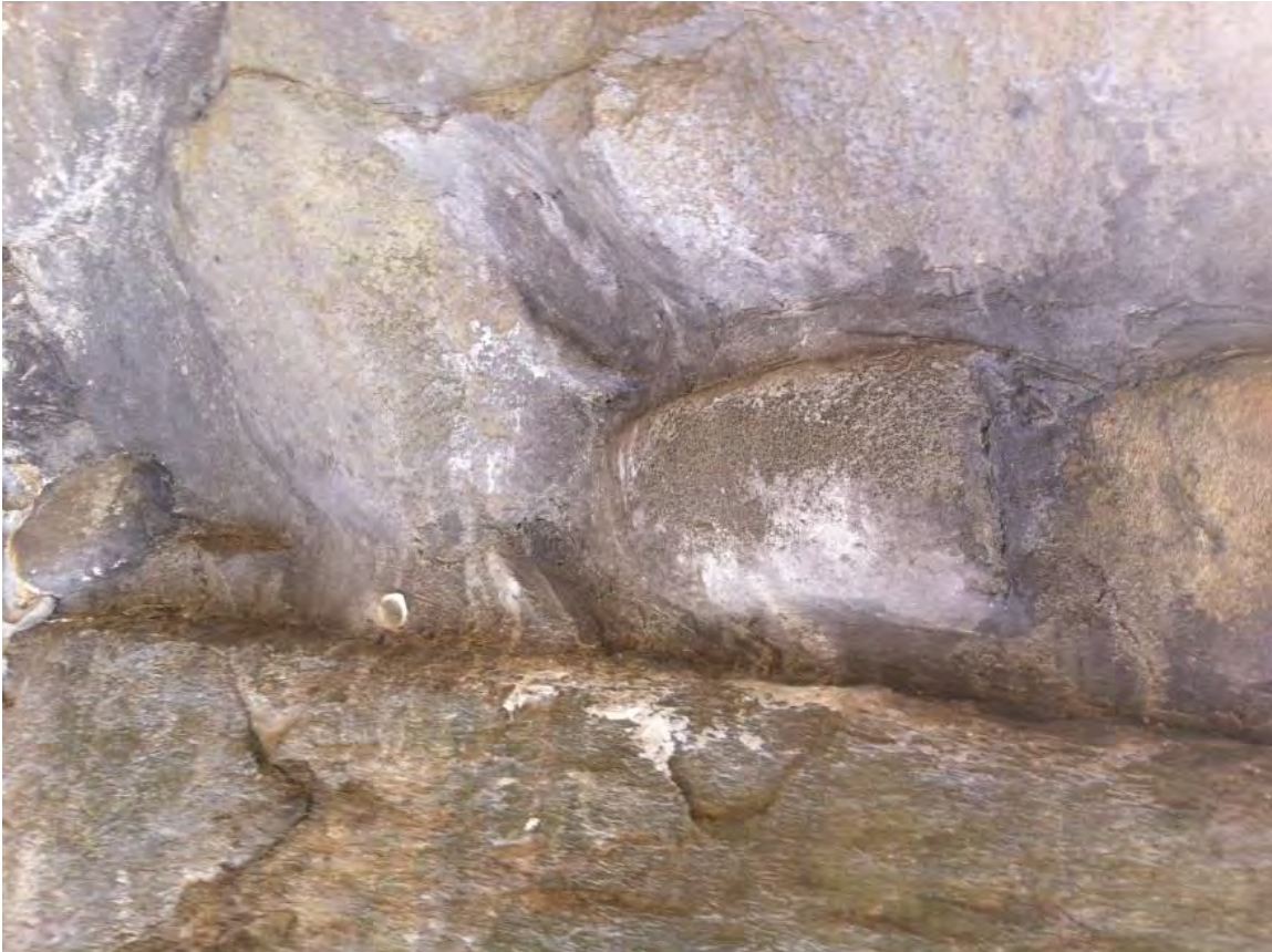
Figure 18 Up-close view of white powdery residue on mortar (VTrans 2013)
