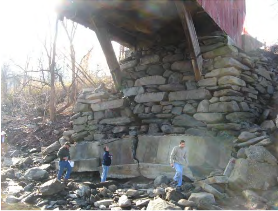
Figure 8 Westerly abutment partially collapsed (VTrans 2011)
