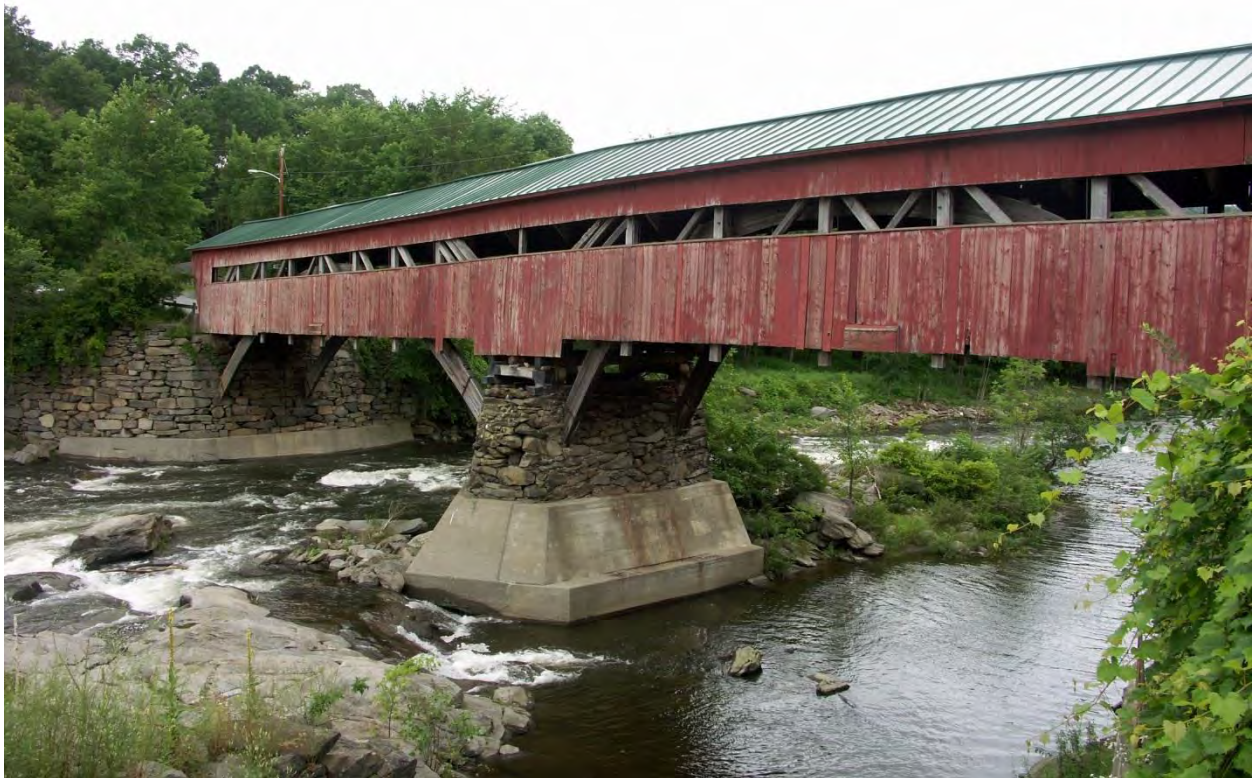
Figure 2 The Taftsville Covered Bridge in 2006 showing the Pier and Abutment that were preserved ( cmh2315fl )
