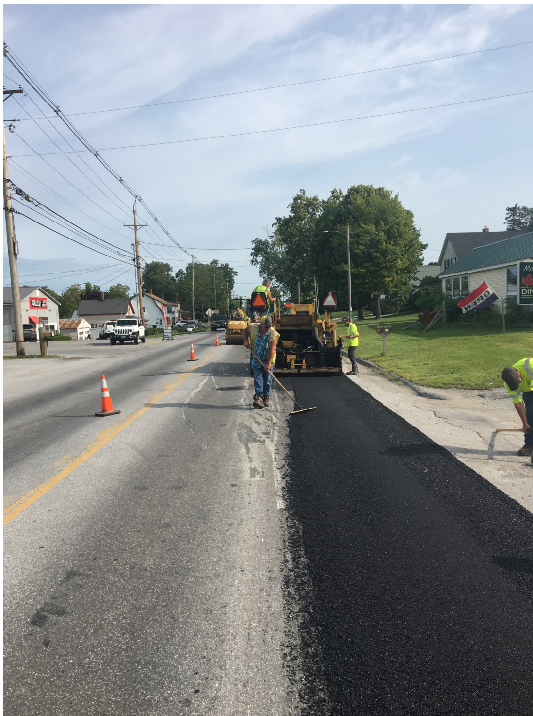
District 8 hot mix patching along a stretch of US 7 in St. Albans
