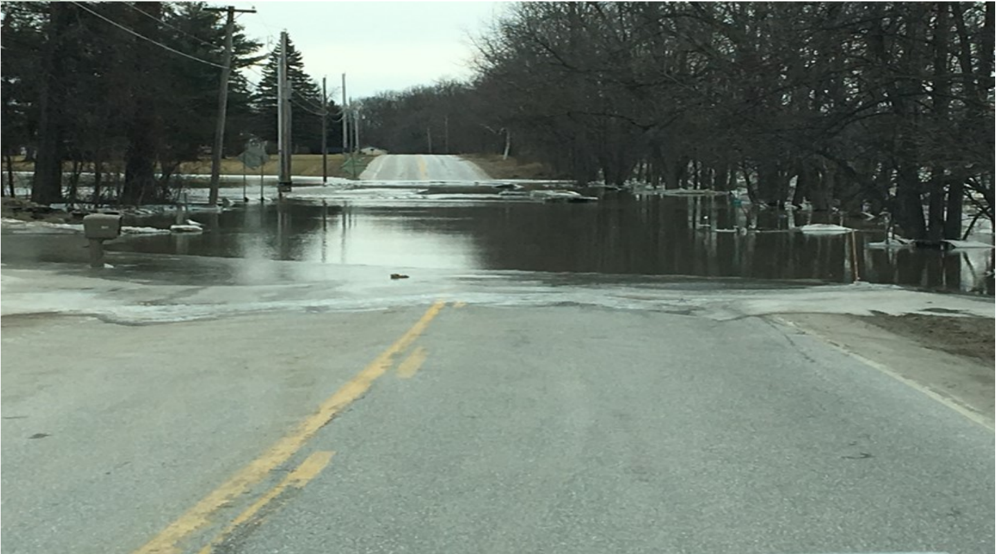
February - Route 78 Swanton, flooding along the Mississquoi River
