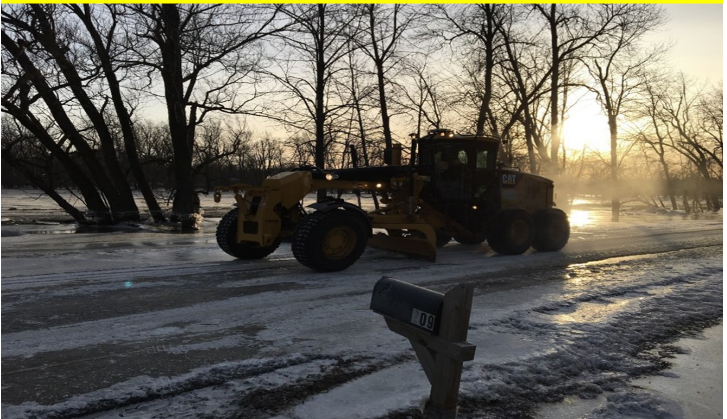
February - Route 78 Swanton, flooding cleanup
