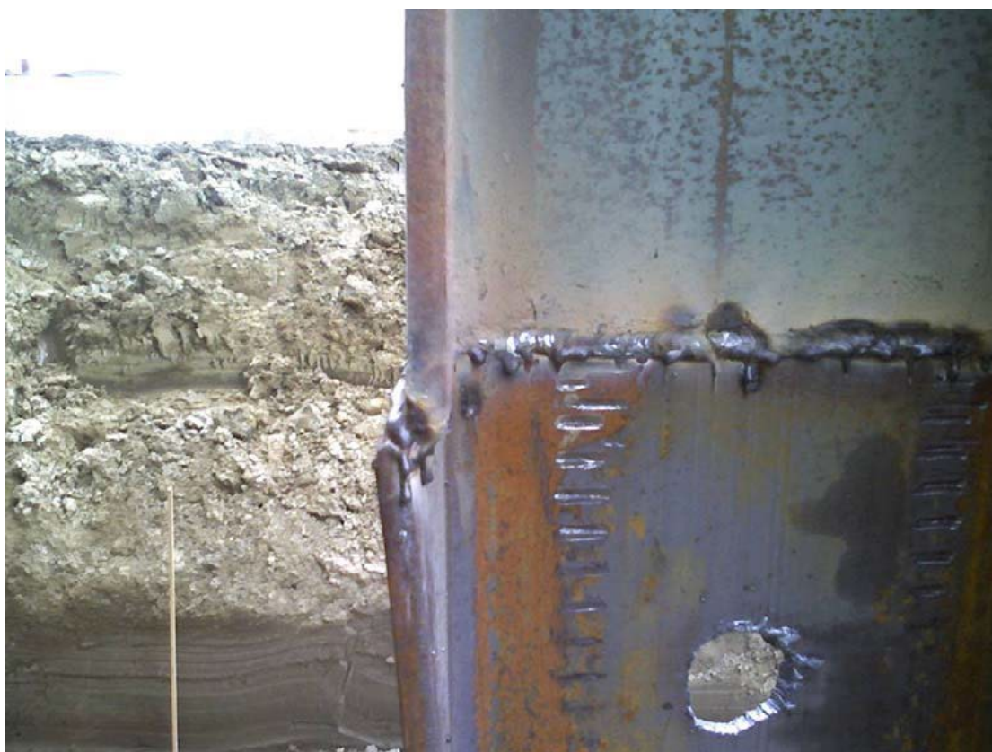
Misalignment, unacceptable profile, slag.
