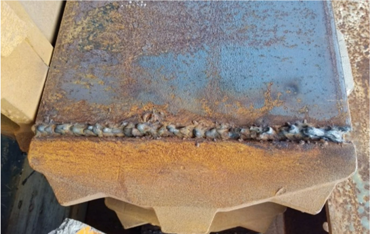
Underfilled joint, lack of fusion, unacceptable profile
