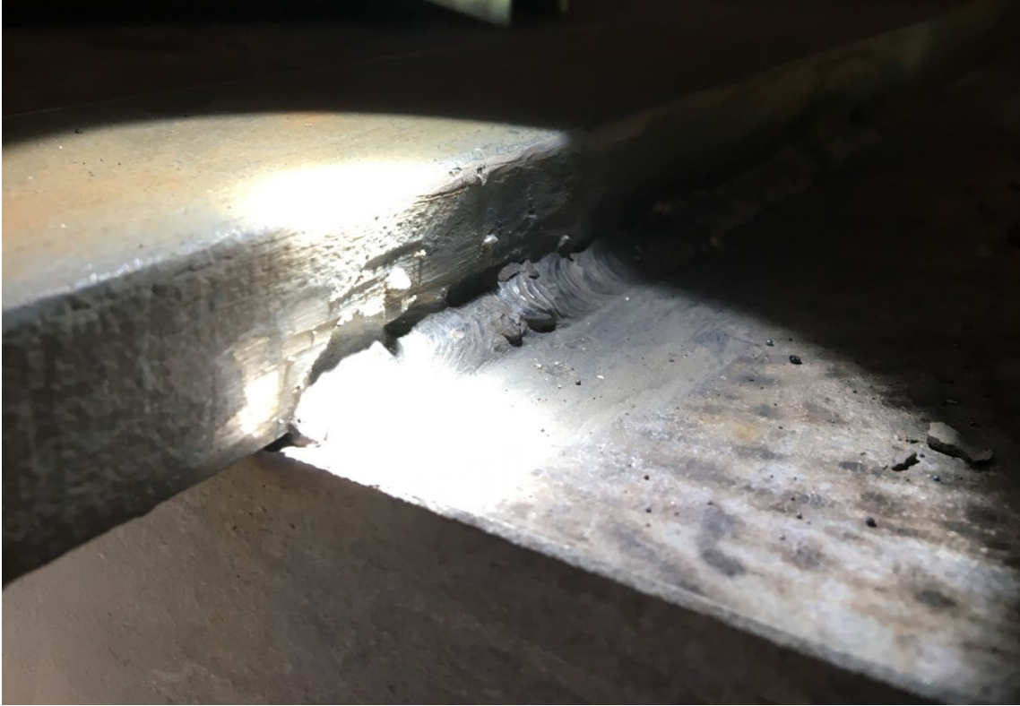
Severe undercut on flange edge welded to sole plate
