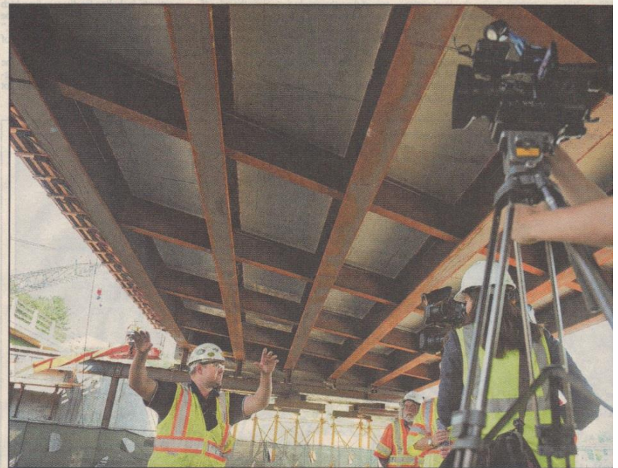
Jeremy Mackling, project manager at PCL, explains the construction of the new Interstate 91 bridges over Route 5 in White River Junction during a news conference at the site last week. The "slide-in" of the interchange bridge is scheduled for this weekend. VALLEY NEWS
