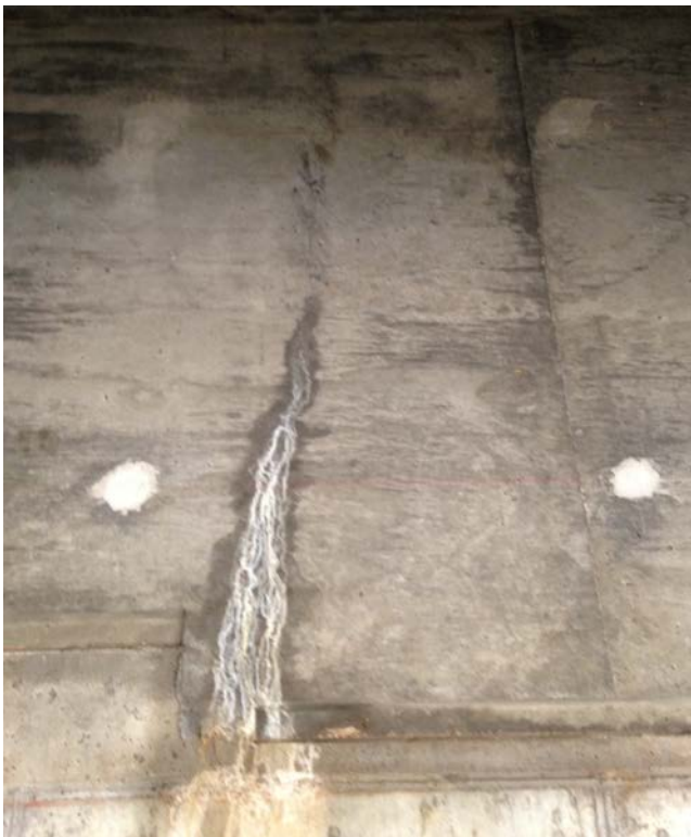
Vertical cracking between integral abutment beams above bridge seat
