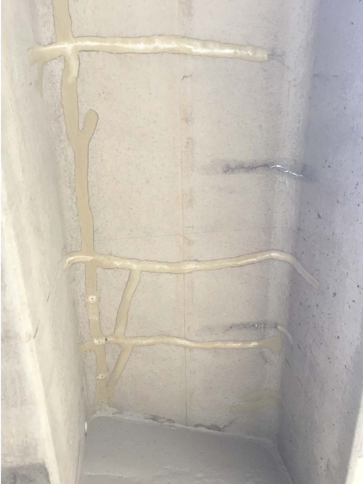
Cracking in NEXT F Section that was repaired at the Fabrication Plant but has opened back up.
