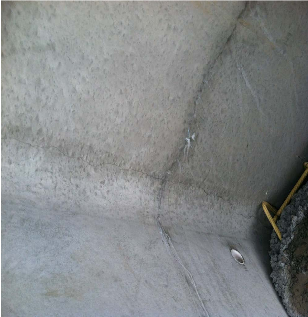
Cracking in flange and web section of NEXT F Beams
