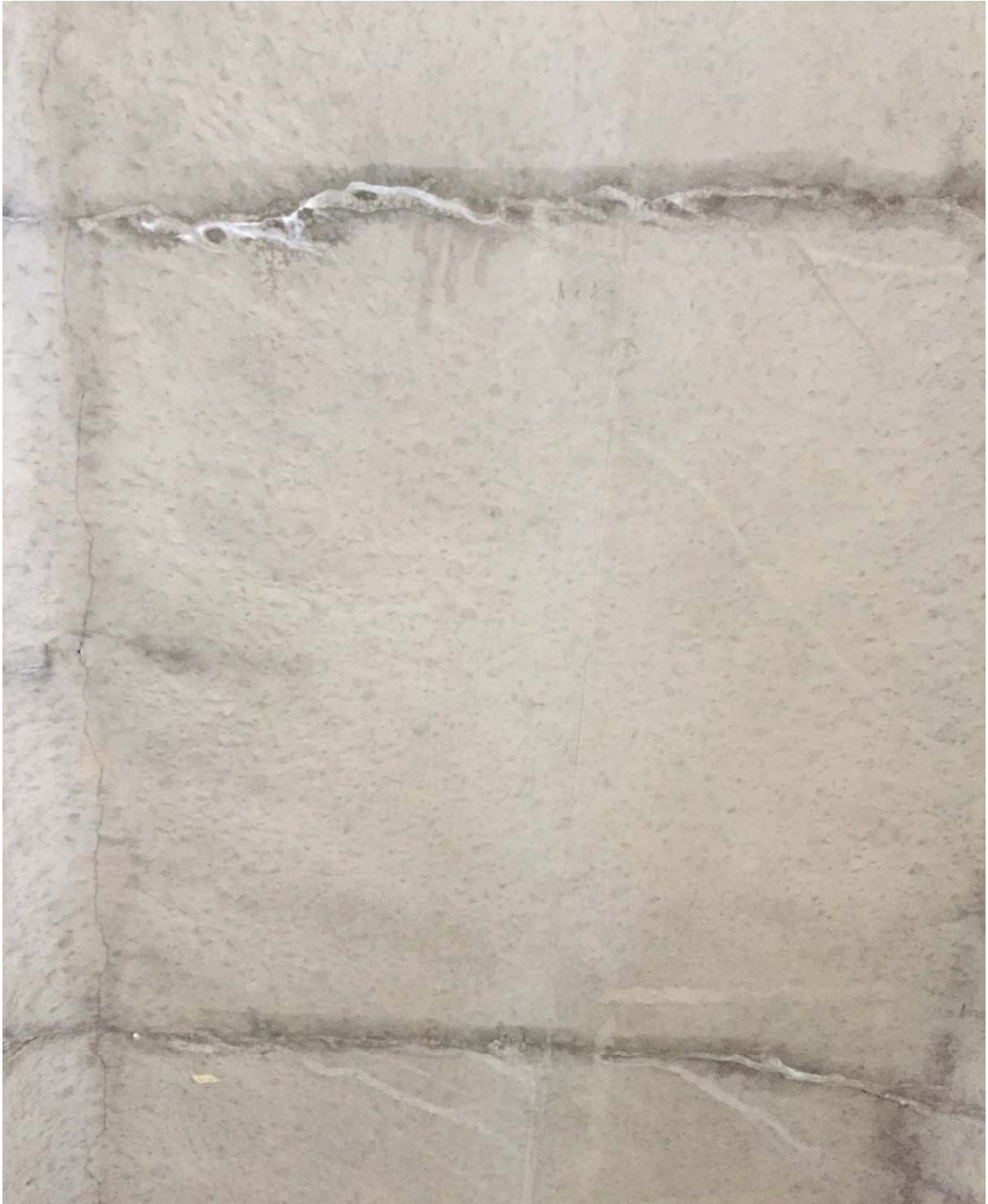
Transverse cracking in NEXT F flange and cracking along the flange to web transition.
