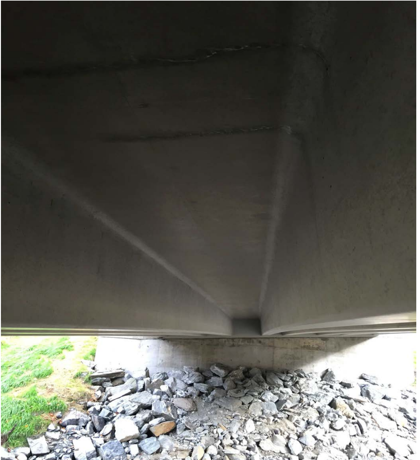
Cracking in flange and web section of NEXT F Beams
