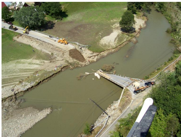
Figure 3: Bridge 19 following Tropical Storm Irene
