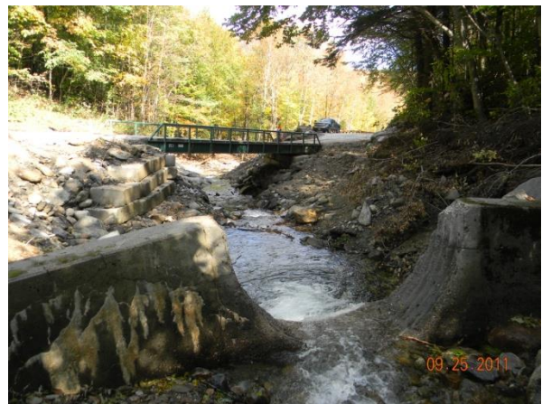
Figure 2: Bridge 13 following Tropical Storm Irene
