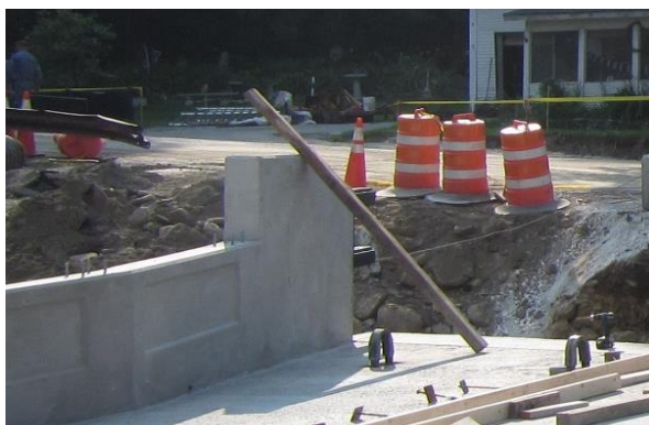
Figure 4: Precast Flare for Historic Rail
