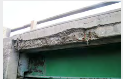
Deck Fascia Deterioration
