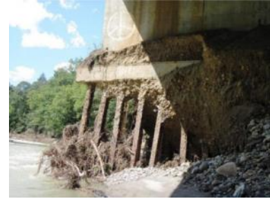
Foundation scour (Dummerston, VT)
