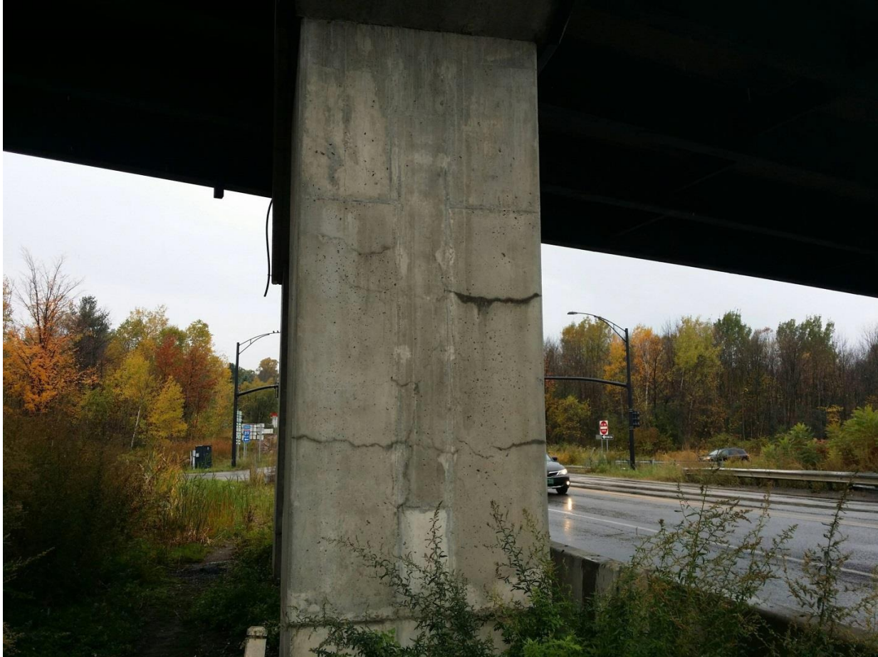
Figure 5.19 Encasement repaired column on Williston I-89 Overpass Tafts Corner, with visible cracking
