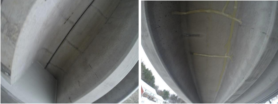
Figure 38: Underside of Concrete Deck. Left Image: shows cracks going at the way through concrete deck. Cracks are highlighted by red ovals. Right Image: sealant used to seal large cracks.
