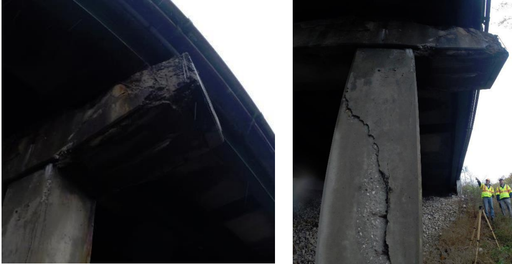
Figure 22: Spalling on end cap and a large crack on end column
