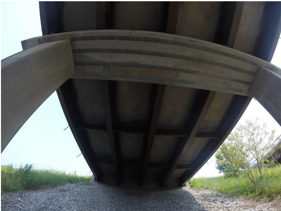
Figure 5.2 Swanton I 89 overpass bridge with FRP strengthening strips bonded to the pier cap, bonding bolt pattern is discernable.
