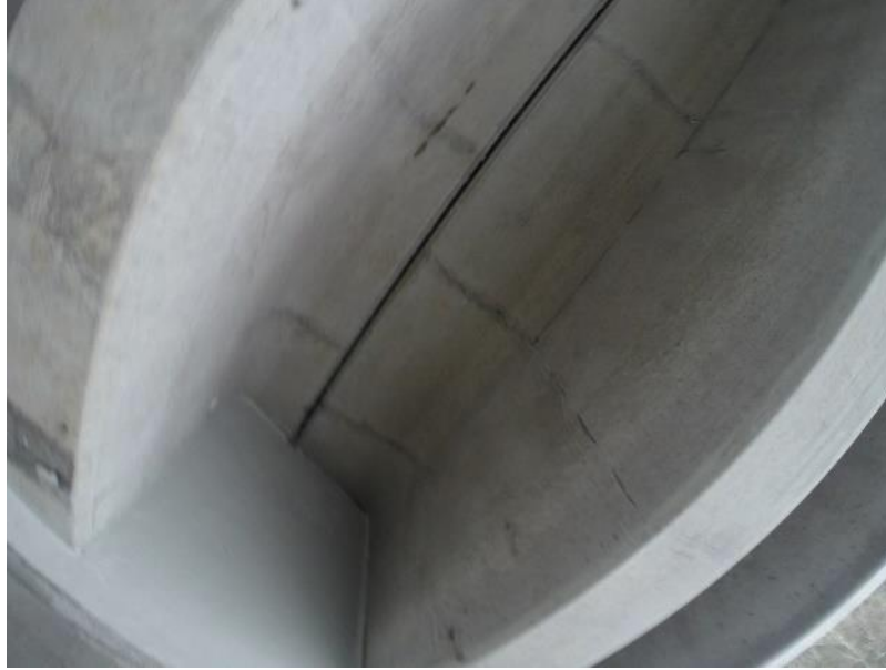
Figure 5.43 Girders have multiple cracks in top flanges, Stowe Rte 100 Gold Brook Crossing Bridge
