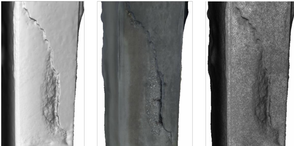
Figure 5.15 Various 3-D photogrammetric renderings of distress column on Colchester/Milton I-89 Bridge
