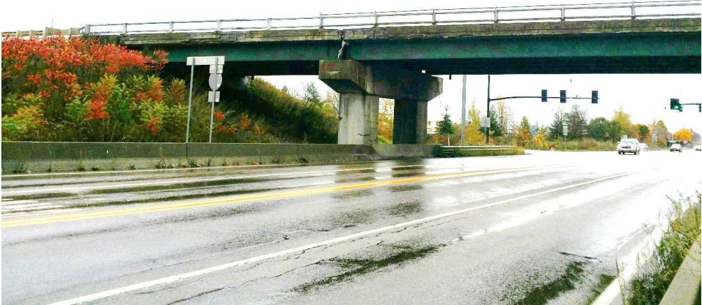
Figure 5.21 Williston I-89 Overpass Tafts Corner with encasement repair of the pier, failed expansion joint gutter and distressed fascia
