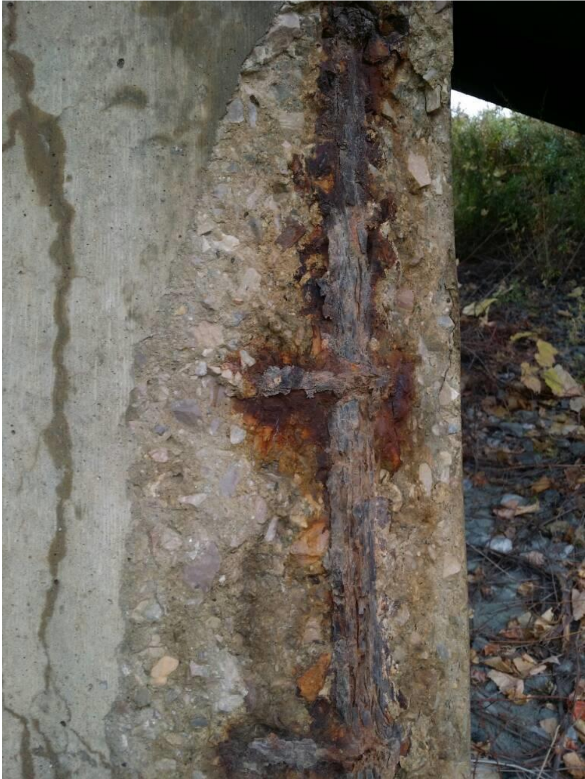
Figure 5.30 Close-up of a distressed column on Richmond I-89 US 2 Underpass Bridge
