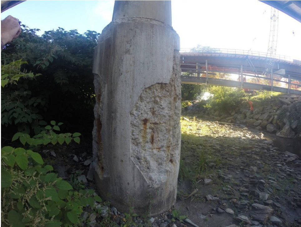
Figure 5.45 End view of pier base with damaged concrete removed on I-89 Waterbury Overpass Bridge
