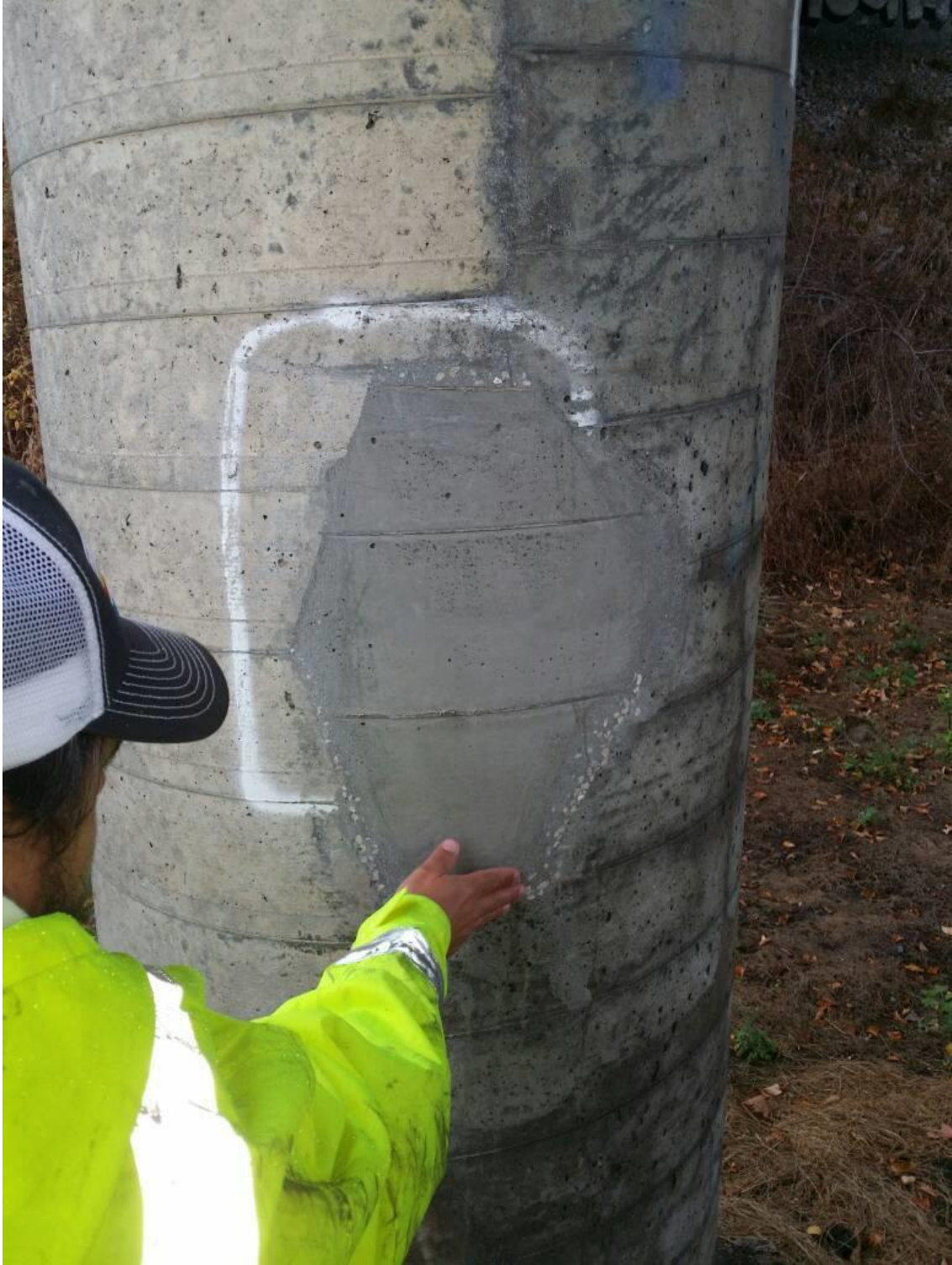
Figure 5.23 Small column patch repair #1 on Williston I-89 Oak Hill Rd Underpass Bridge
