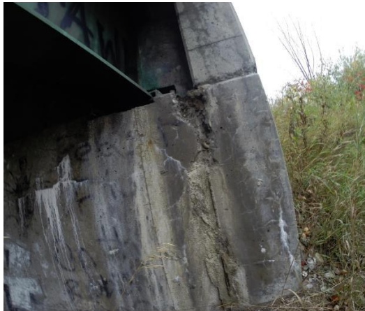
Figure 29: Scaling on abutment around bearing and beam
