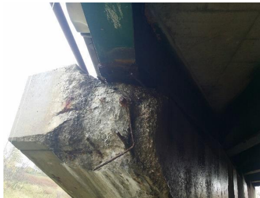
Figure 34: End cap spalling and steel corrosion with non-existing bearing.
