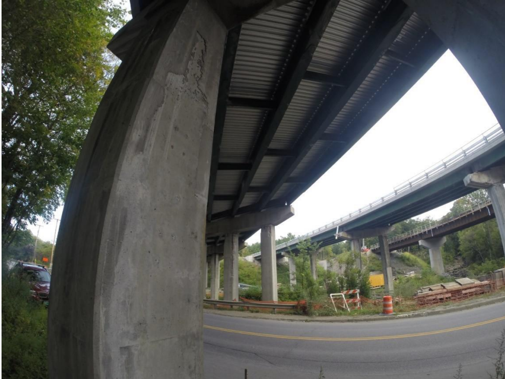
Figure 5.50 Pier on I-89 Waterbury Overpass Bridge with patch repairs, note the extended gutters on span in background
