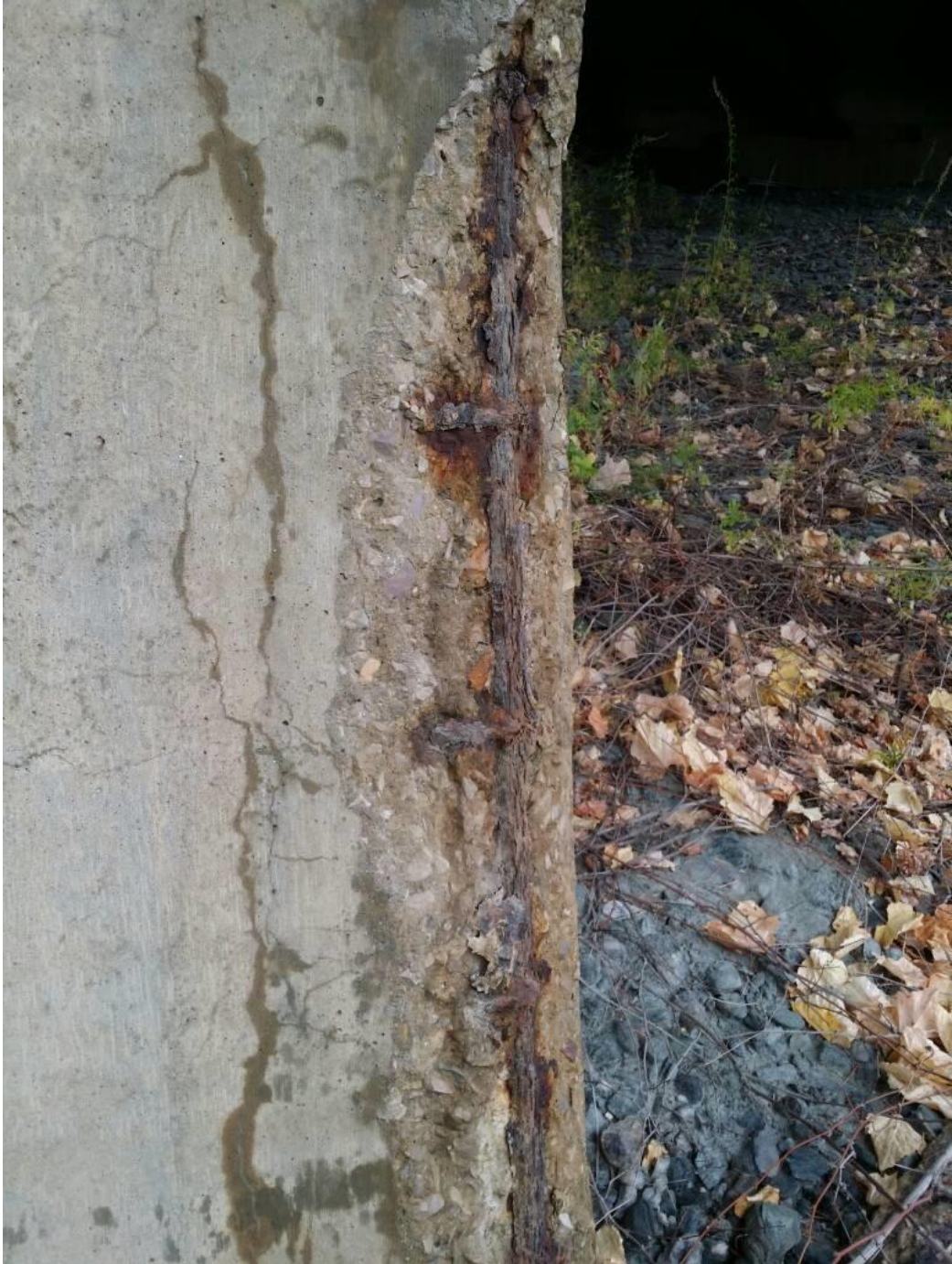
Figure 5.29 Distressed column on Richmond I-89 US 2 Underpass Bridge
