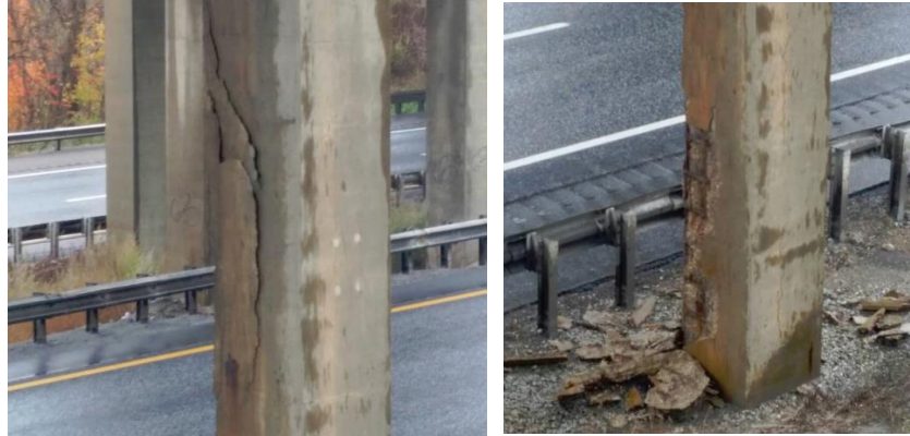
Figure 33: Spalling and steel corrosion on concrete column. Notice concrete fragments falling near road.
