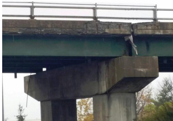
Figure 27: Spalling and steel corrosion on concrete fascia.
