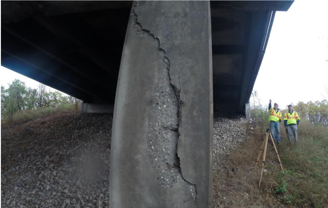
Figure 5.14 Column with distress on Colchester/Milton I-89 Bridge
