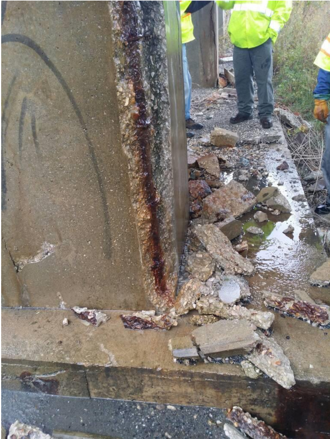
Figure 5.33 Square column with spalling at the corners on Richmond I-89 US 2 Underpass Bridge
