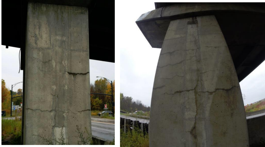
Figure 26: Possible dry shrinkage cracks on concrete column that has had a 6" thick concrete jacket around column.
