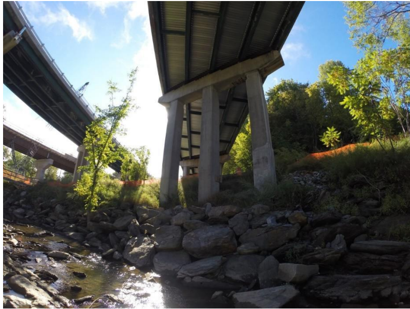
Figure 5.52 Repaired pier on I-89 Waterbury Overpass Bridge with patch repairs, note the use of integrated corrugated panels on new concrete deck.
