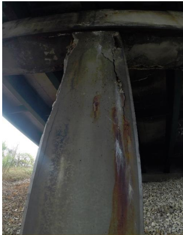
Figure 21: Other side of middle column. Notice Spalling, cracks and corrosion stains.
