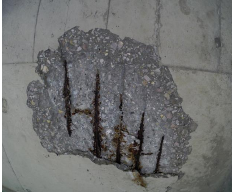
Figure 5.27 Underside Deck Spalling on Williston I-89 Oak Hill Rd Underpass Bridge
