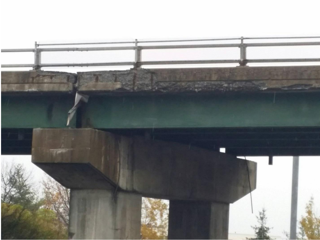
Figure 5.22 Closeup of Williston I-89 Overpass Tafts Corner with encasement repair of the pier, failed expansion joint gutter and distressed fascia
