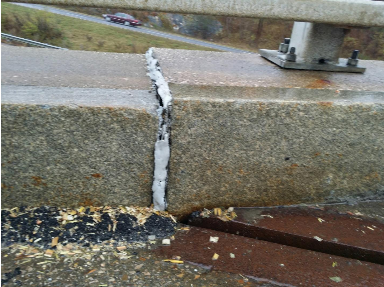
Figure 5.40 Subsided bearing leading to vertical misalignment of expansion joint on Richmond I-89 US 2 Underpass Bridge
