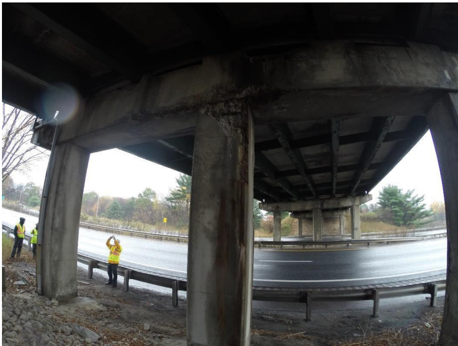
Figure 19: Column and cap Spalling and steel corrosion
