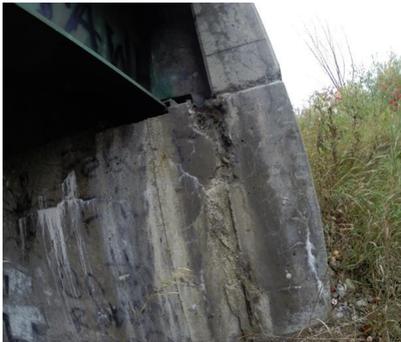
Figure 5.28 Scaling on Abutment and Beam on Williston I-89 Oak Hill Rd Underpass Bridge
