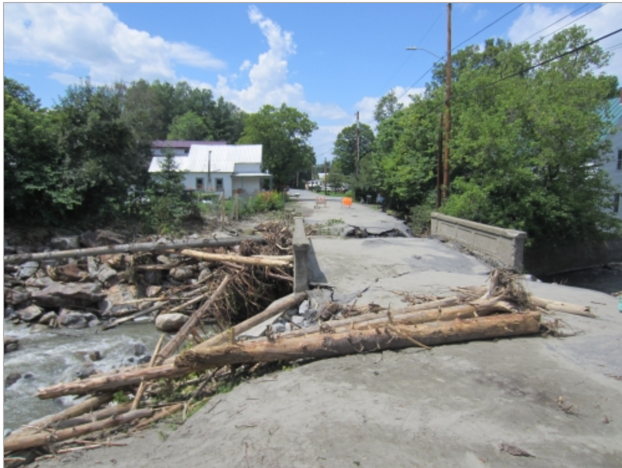
Figure 5 Damage to Infrastructure from Great Brook at Mill Street in July 2015
