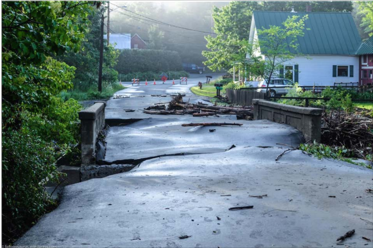
Figure 1 Damage caused by debris blockage of a crossing structure
