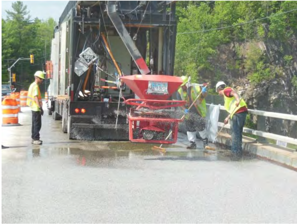
Figure 3. Installation of Flexogrid. Epoxy has been squeegeed on and the aggregate is being spread on the surface.
