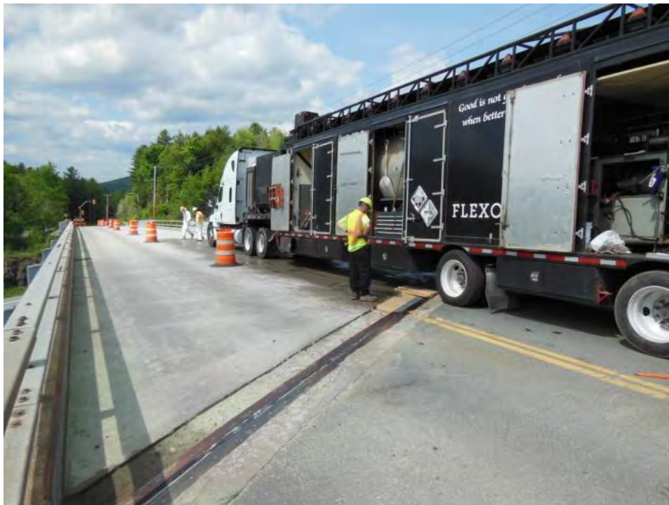
Figure 2. Poly-Carb installation vehicle, and the prepared condition of the concrete bridge deck.
