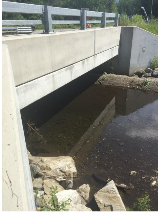
Figure 2: Overall View of Bridge 165 on VT 100, Warren VT. Right side of bridge facing south
