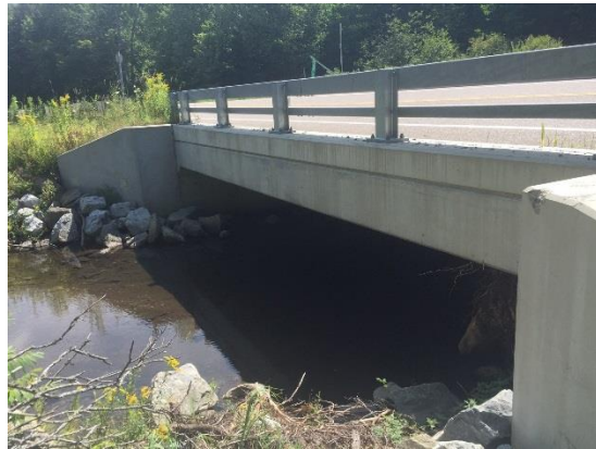
Figure 3: Overall View of Bridge 165 on VT 100, Warren VT. Left side of bridge facing north
