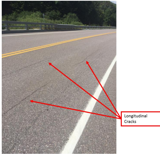
Figure 6: Longitudinal cracks on northbound lane
