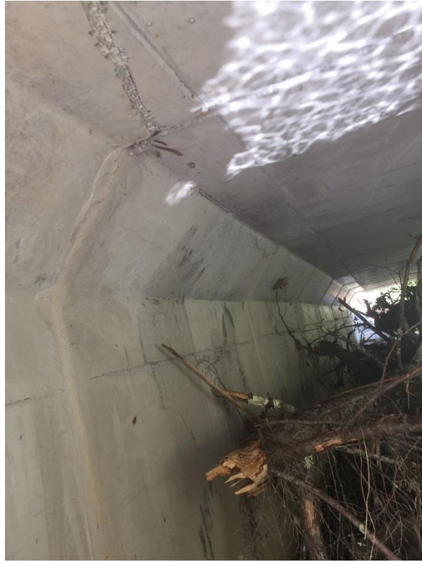
Figure 8: Bridge underside with debris
