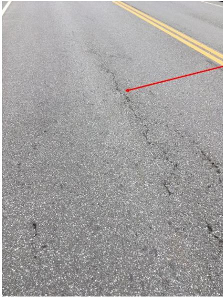
Minor Transverse Cracking in Northwest bound travel lane
