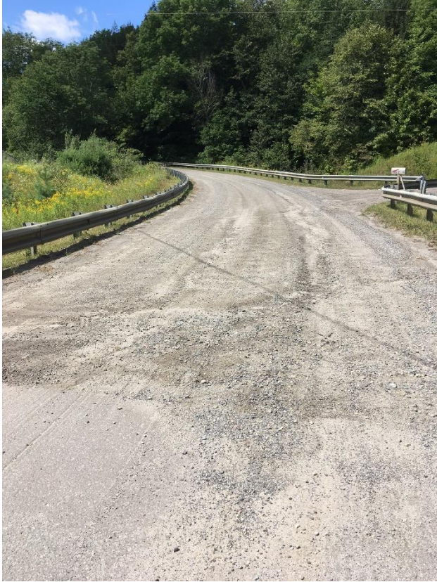
Some potholing and washboarding was noticed on the west end approach of Bridge 89.
