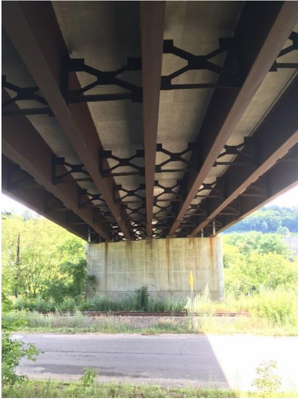
Full view of the underneath of the Bridge 1, near the west abutment looking towards the east bridge abutment.
