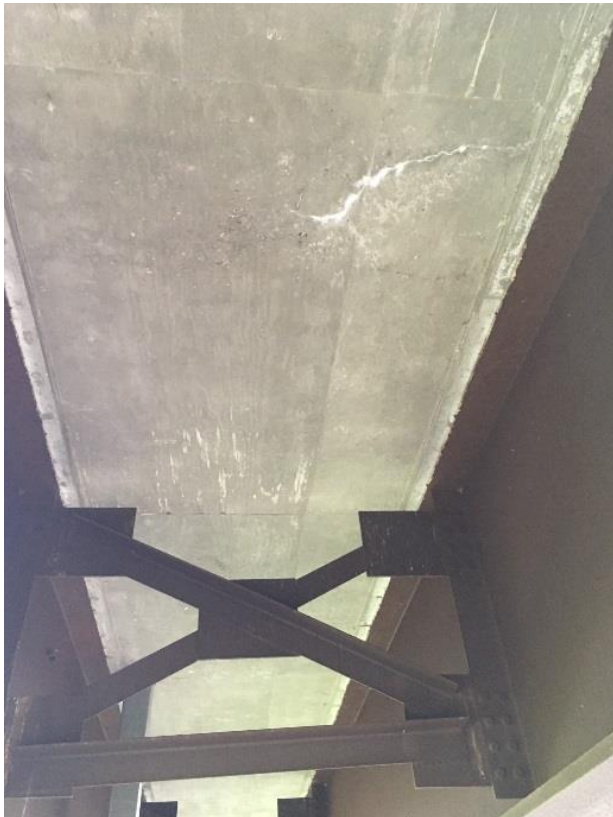
No new cracking or deterioration was visible on the underside of Bridge 86. A white substance was found protruding from what seems to be a crack in a concrete deck slab. No moisture was present along the crack making it likely that the white substance is either evidence of the Eliminator membrane sealing a prior concrete deck crack during the application of the membrane or the leaching of calcium from the concrete structure, a sign that the concrete is degrading and deteriorating. A closer inspection of the crack would have to be conducted to determine whether it's one or the other.
