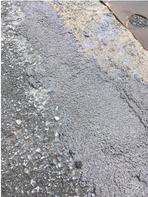
A close-up of the patching around the bridge joint on the west side of Bridge 1.
