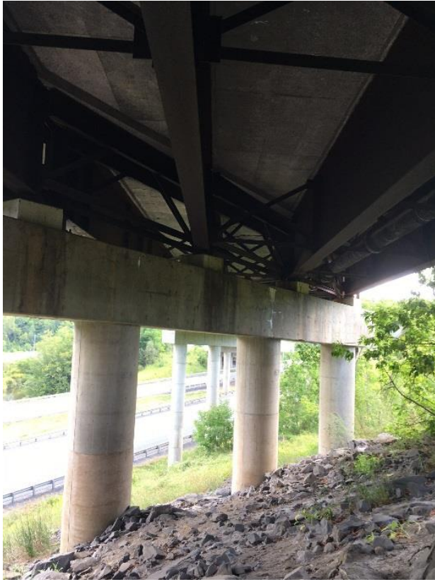
Full view of the underneath of Bridge 86, near the Northwest abutment looking towards the Southeast end of the bridge.
