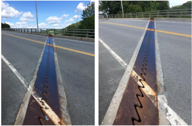
The photo on left shows the bridge joint on the Southeast end of the bridge, while the photo on the right shows the bridge joint on the Northwest end of the bridge. Both the Northwest and Southeast bridge joints were in excellent condition, where little to no deterioration is evident.
