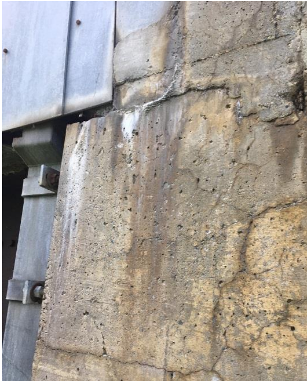
Bridge abutment cracking and deterioration on the West side of Bridge 1.
