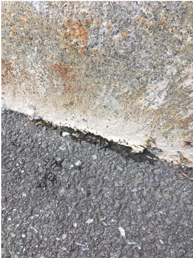
The bridge curb shows overspray (white) that occurred during installation of the Eliminator membrane.
