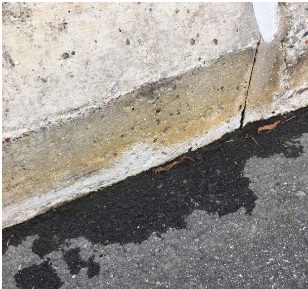
The bridge curb shows overspray (white) that occurred during installation of the Eliminator membrane.
