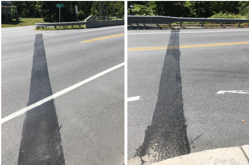
The photo on the left shows the bridge joint on the east end of the bridge while the photo on the right shows the bridge joint on the west end of the bridge. The bridge joints were in good condition.
