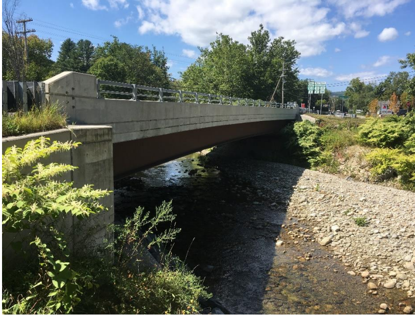
Side view of Bridge 9 on VT 103, from the east end looking to the west.
