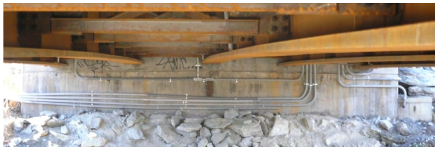
Figure 3-2: Cable Routing on the Abutment
