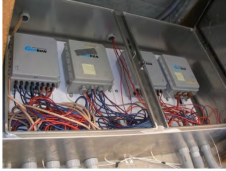
a) Multiplexers at Abutment
