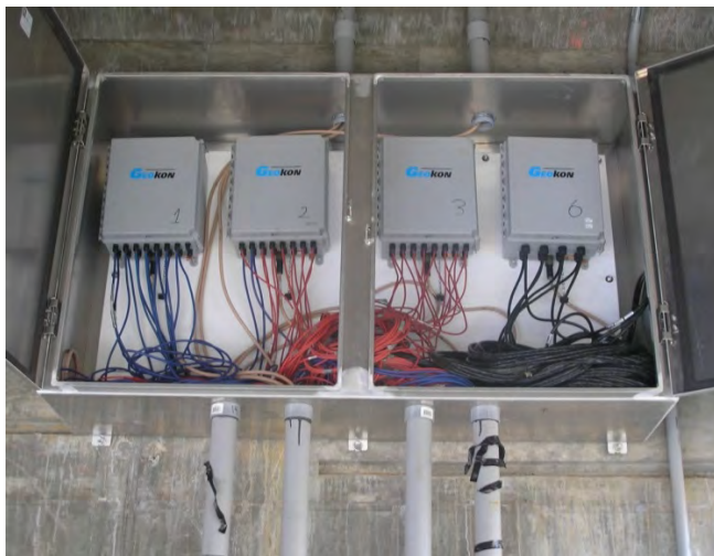
a) Multiplexers at Abutment
