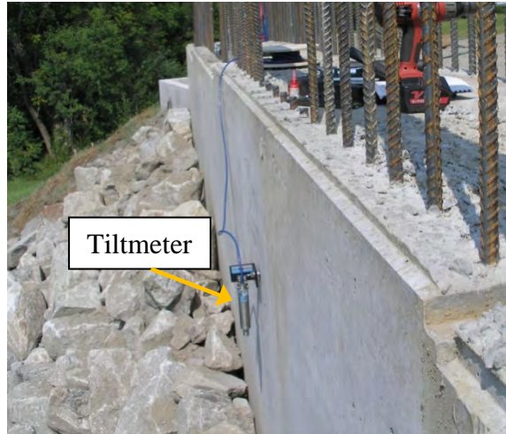
Figure 3-50: Tiltmeter Location Abutment at East Montpelier Bridge
