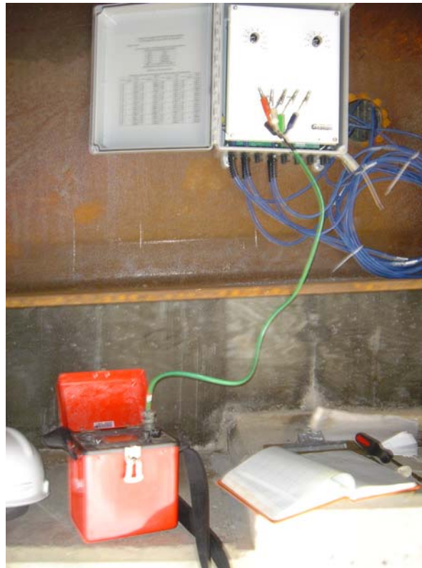
Figure 5.6. Central Breaker Box and Geokon GK-403 Vibrating Wire Readout Box.
