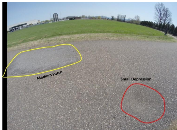
Figure 48 Test Spot with Medium Asphalt Patch and Small Asphalt Depression
