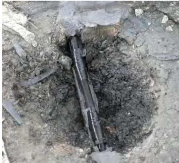
FIGURE 3 Holes after LED removal.
