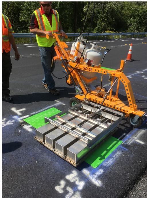
Figure 1: Ennis-Flint Representative Jeremy Crow showing L & D Crew how to Operate the StreetHeat SR-28
