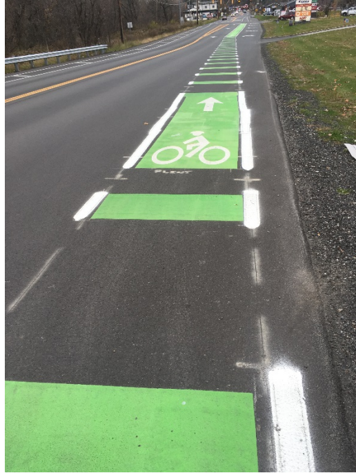
Figure 12: PreMark Bike Lane Blocks at Price Chopper Intersection with added Polyurea White Marks
