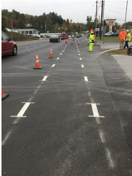
Figure 29: Bike Lane near CVS Before Transpo Color-Safe was Installed
