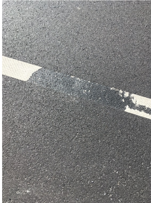
Figure 44: Brite-Line HDX Inlaid Tape Failure at 9+50 on Westbound Side
