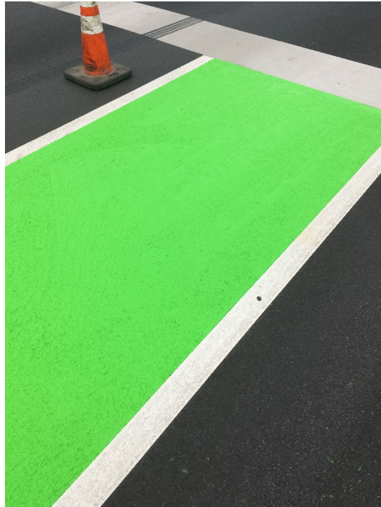
Figure 31: Close-up of the Solid Section of Transpo Color-Safe at CVS Intersection when Finished
