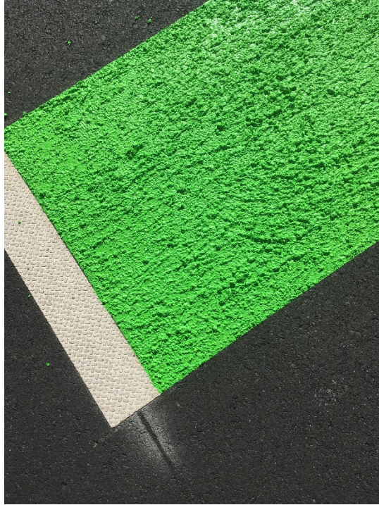
Figure 42: Close-up of a Transpo Color-Safe Bike Lane Block Near VW Dealership
