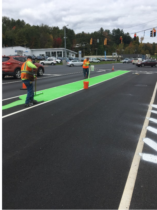
Figure 32: Application of Transpo Color-Safe at CVS intersection and Removing of Painters Tape
