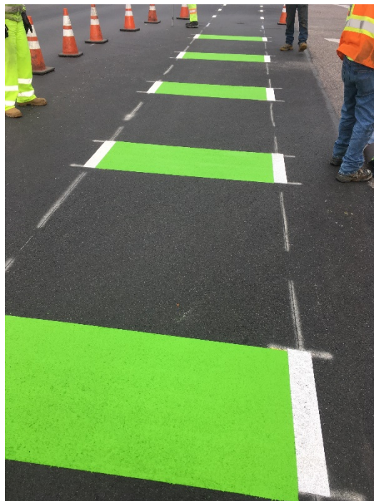
Figure 16: Curing CycleGrip MMAX from one kit at the Vermont Shopping Center Intersection
