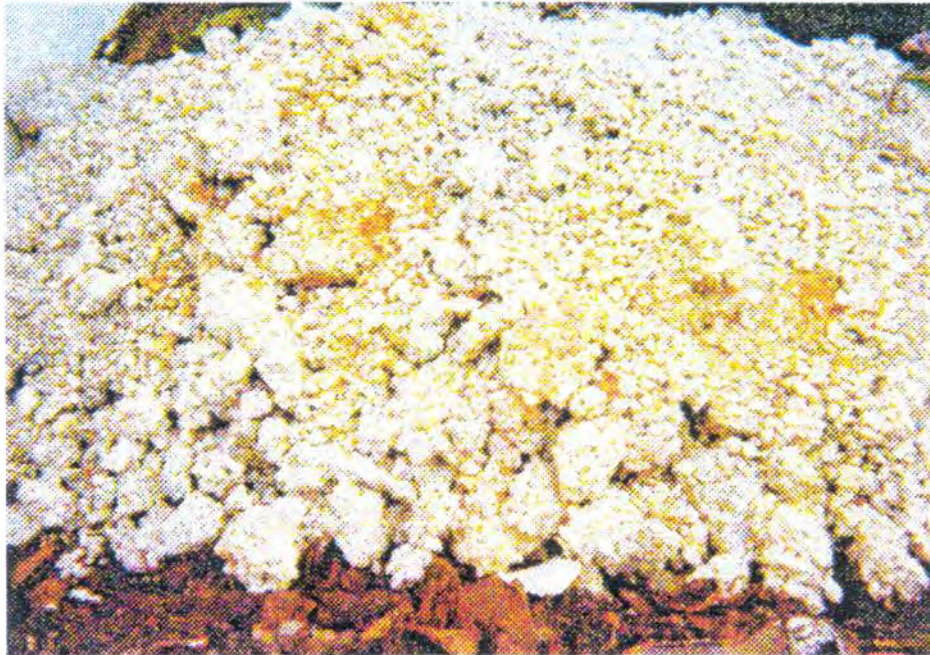
Cement-treated base course mixed at Heindel and Noyes' North St. facility, using washed stone aggregate purchased from Hinesburg Sand & Gravel, Hinesburg, VT
