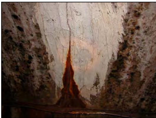
Figure 1 – Cracked in Richmond, 08/26/03
