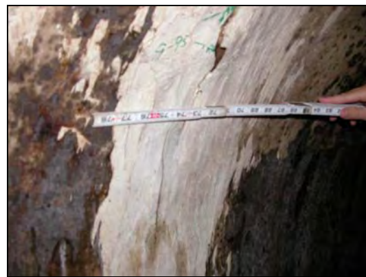
Figure 2 – Patching in Richmond, 7/2/07
