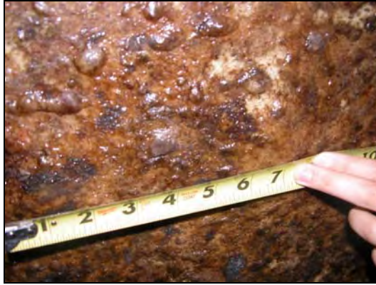
Figure 3 – Blistering in Addison, 6/20/06
