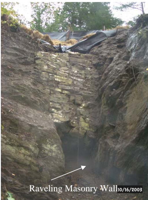
Figure 7: Masonry wall below washout.
