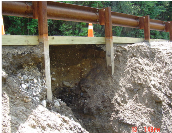
Figure 1: Undermining of north side of VT 73 in Forest Dale.
