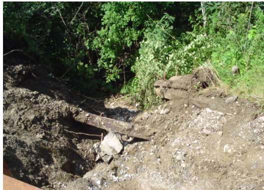
Figure 2: Washout of timber cribbing above mortared masonry wall. (View from road level)
