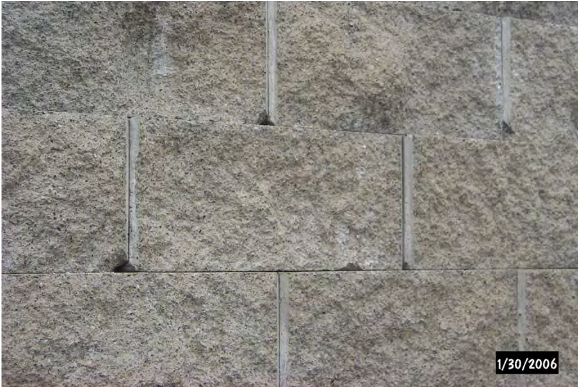
Figure 9 – Blocks with chipped corners
