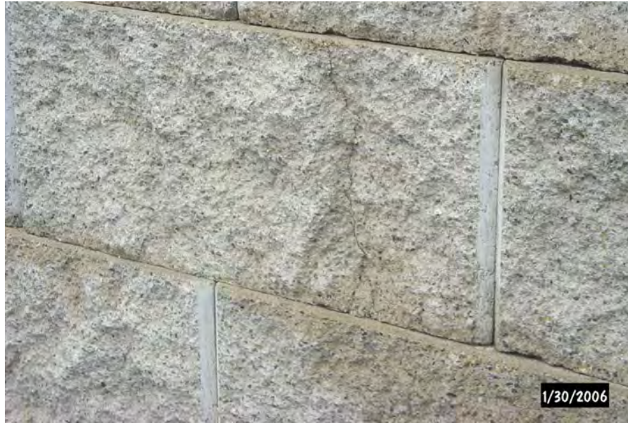
Figure 8a – Vertical fracture
