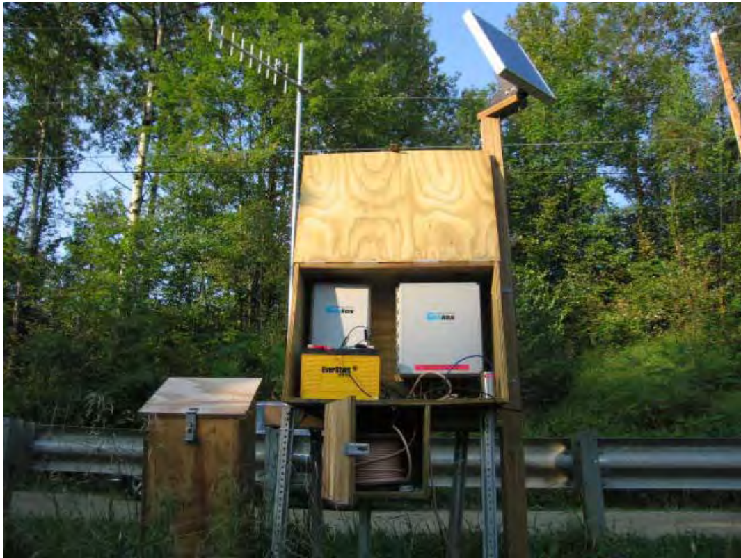
Figure 3.10 View of the data acquisition system when the protective box is open. The battery is in the front left, the multiplexer behind, and the datalogger to the right. The cell phone antenna is in the upper left and the solar panel in the upper right.
