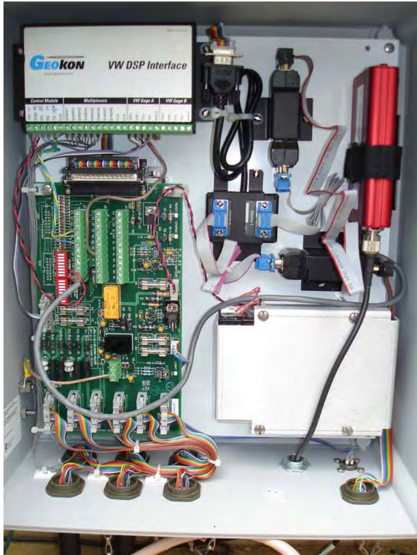
Figure 3.9 Geokon Micro-10 datalogger.
