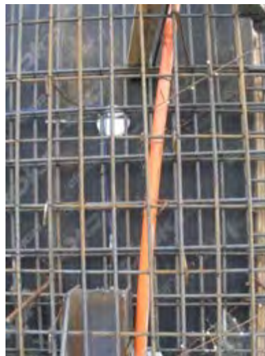
Figure 3-54: Inclinometer Casing Route around the Girders at the Top
