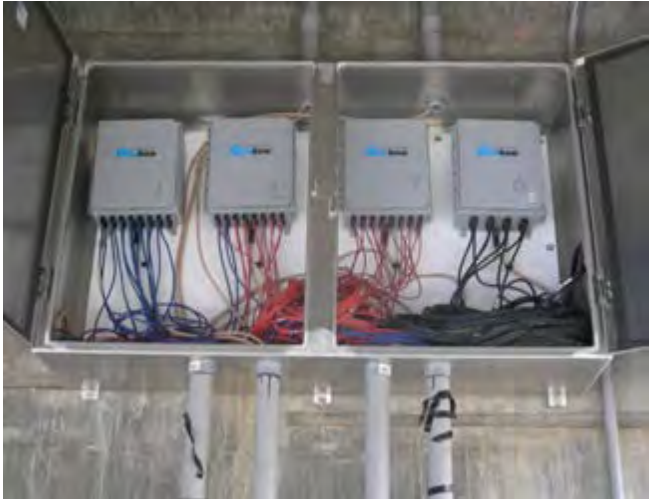
a) Multiplexers at Abutment
