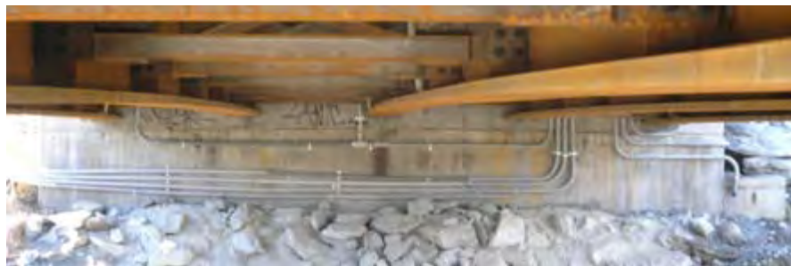
Figure 3-2: Cable Routing on the Abutment
