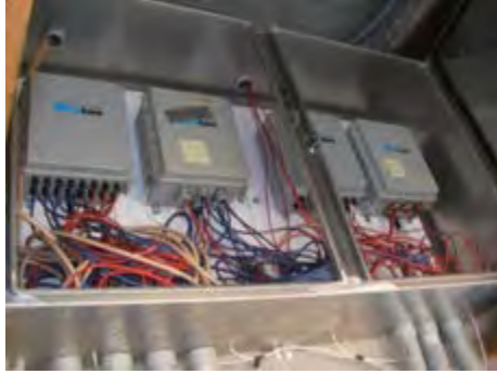
a) Multiplexers at Abutment
