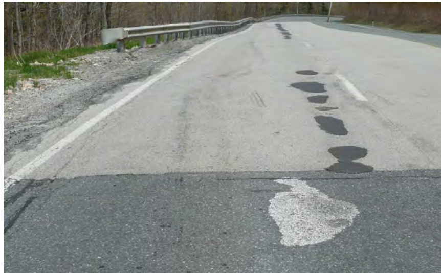
Figure 21 Pothole repair less than a year after application.
