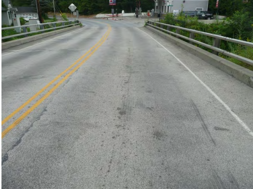
Figure 18 The darken wheel paths show where the aggregate has been stripped, exposing the underlying epoxy (2010).
