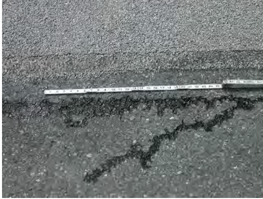
Figure 12: Water leaking from the centerline joint
