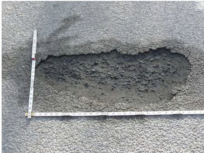
Figure 14 An example of a pothole. The underlying pavement was lifted out with the overlay.
