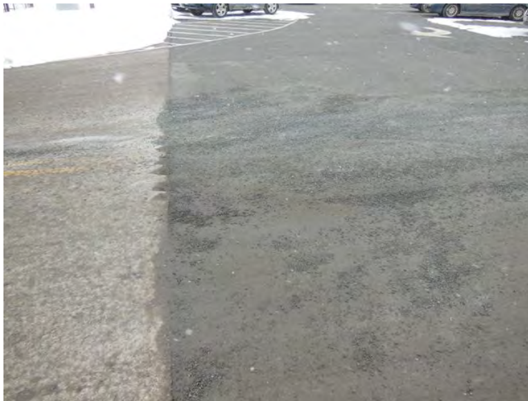
Figure 13. Deterioration at the transition between the bituminous drive (left) and porous concrete lot (right) after five winter seasons.
