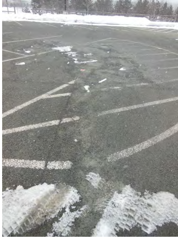
Figure 12. Deterioration in the gore area of the front portion of the lot after five winter seasons.
