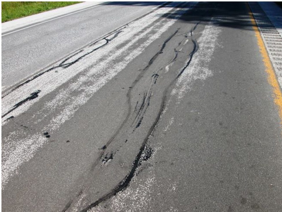
Figure 17: 2007 Crackfill in Slurry Seal section.
