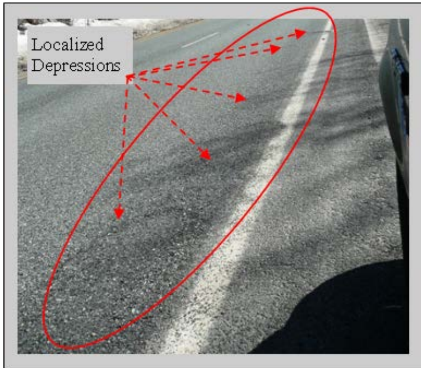
Figure 21: Localized depressions located at MM 44.5 in the travel lane within the NovaChip® section.
