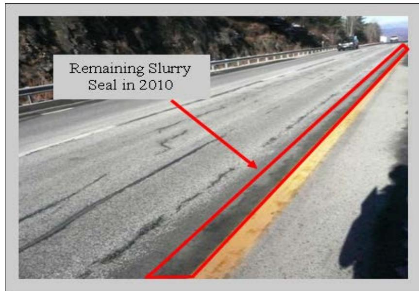
Figure 22: Remaining Slurry Seal Treatment in 2010.
