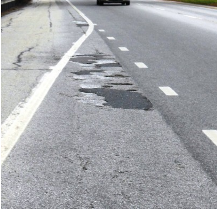
Figure 23: Potholes near Exit 7 in 2013.
