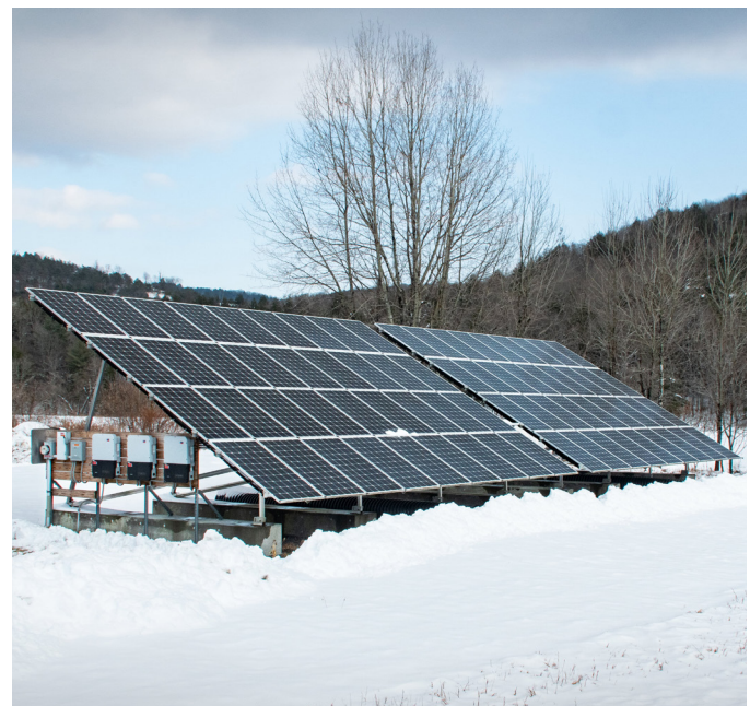
TUNBRIDGE. As the Agency turns to green technologies, one maintenance garage has installed new solar panels and an electric heating system to transition the facilities towards self-sufficiency.
