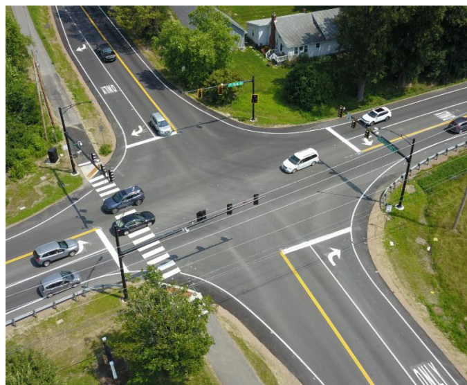
HINESBURG. An intersection improvement project was completed along VT Route 116. Improvements include a widened roadway, new turn lanes, and a new traffic light system to make the flow of traffic safer and more efficient.
