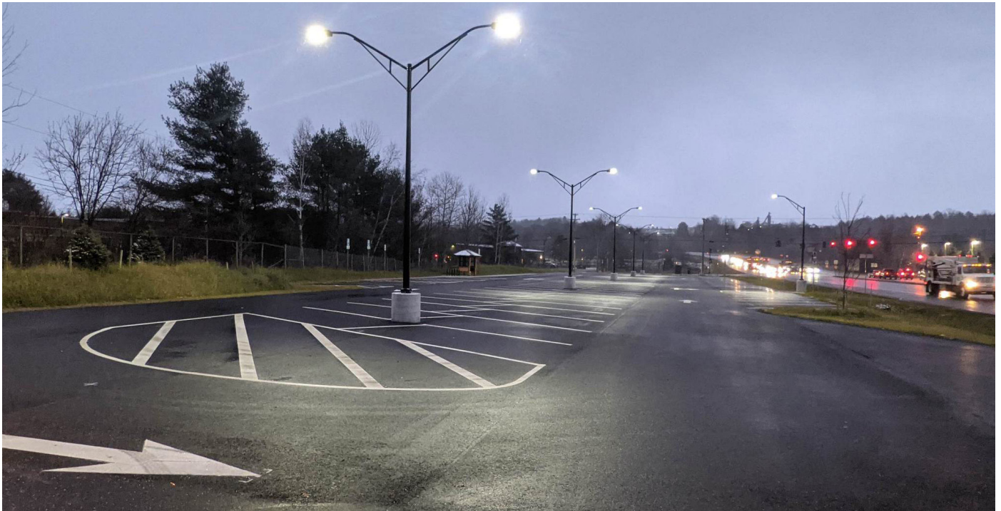
BERLIN. The existing Park and Ride facility at the intersection of VT Route 62 and Paine Turnpike North underwent major improvements this past construction season. The facility was expanded to create more vehicle parking spaces and features all new paving, markings, and lighting systems.
