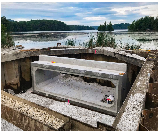
SUDBURY. Closing a roadway for construction can be a challenge for the traveling public. When two culverts needed replacing along VT Route 30, crews used accelerated bridge construction methods to complete the project as quickly as possible. New pre-cast concrete box structures were installed, and the roadway was reopened in three weeks, far ahead of schedule.
