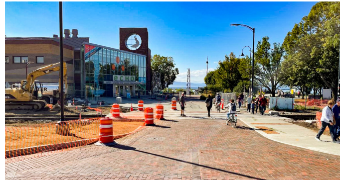
BURLINGTON. Crews were busy throughout 2021 preparing the Burlington Waterfront for the 2022 arrival of AMTRAK services.
