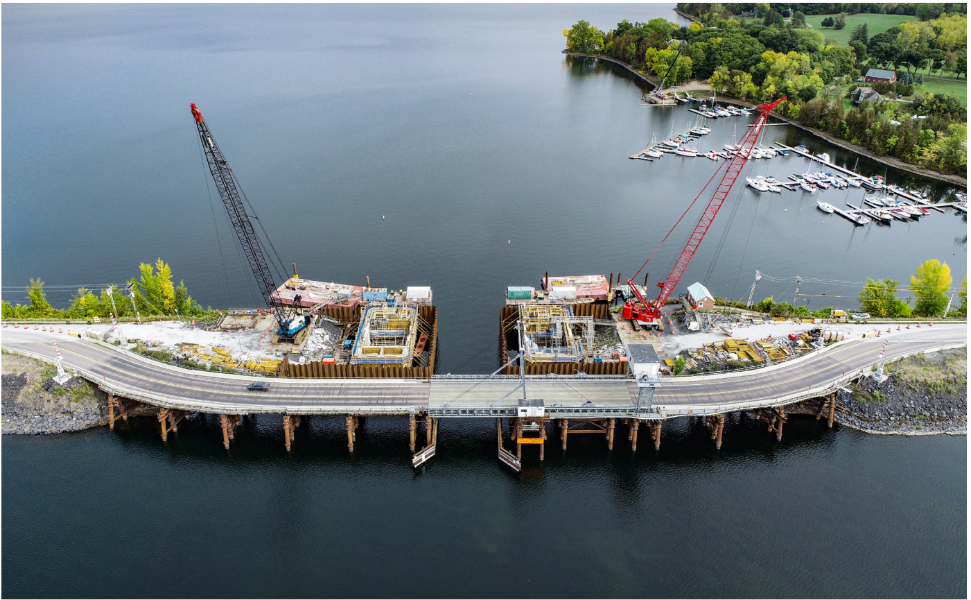
NORTH HERO - GRAND ISLE. The past year brought another busy season of construction on the US Route 2 Drawbridge replacement project. The structural concrete for the new bascule piers was completed as crews began erecting steel and preparing for the installation of the new drawbridge control house.
