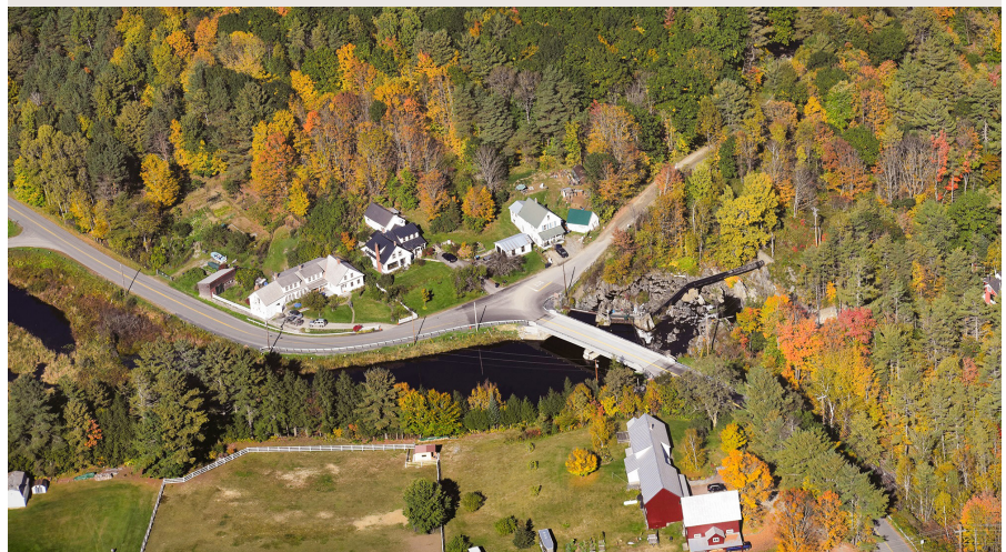
NEWBURY. The Boltonville Bridge over the Wells River connecting US Route 302 and Boltonville Road received a major face lift this past season as crews fully replaced the bridge deck and steel beams. New bridge joints were also installed, along with minor repair work to the concrete substructure. These improvements will increase the longevity of the bridge and will protect the structure from further deterioration due to chlorides.
