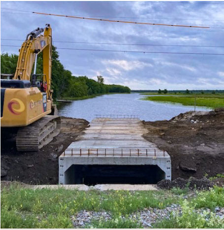
SWANTON. When a washout eroded part of VT Route 78 in late June, AOT crews acted fast and installed a new box culvert in just a few days, enabling this important route through the Champlain Islands to reopen for the Independence Day holiday weekend.
