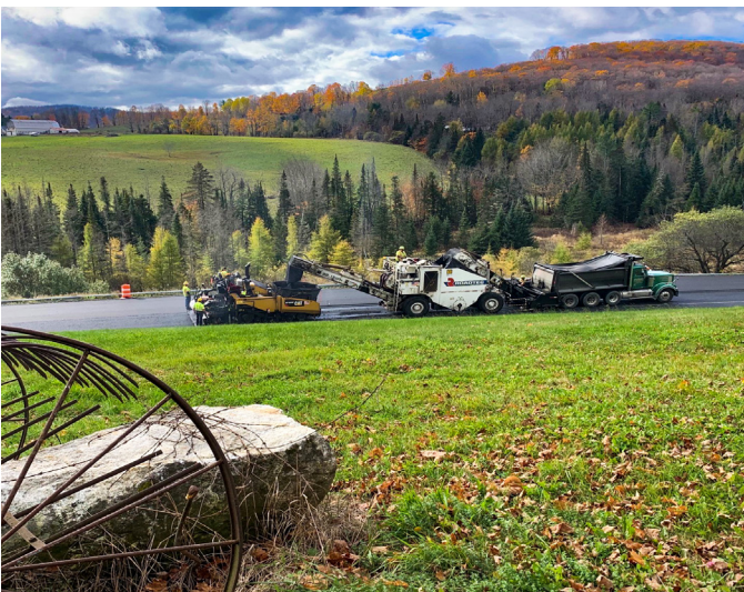
CHELSEA-THETFORD. A 15-mile stretch of VT Route 113 is under a full depth reclamation project. The original roadway was stripped to gravel and then rebuilt, along with ditching, guardrail, and alignment improvements. Paving of the final course is planned for 2022.
