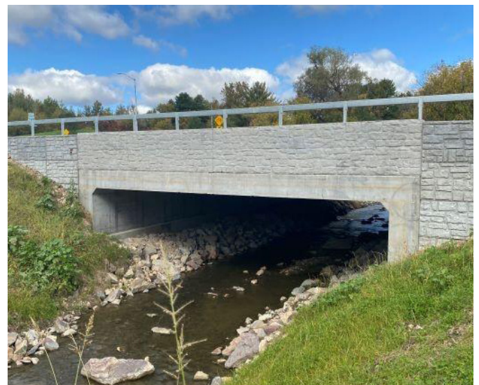
ESSEX. During the summer, a failing metal pipe culvert along VT Route 117 was replaced with a new concrete buried structure and bridge over Alder Brook. The new structure is much wider, allowing for decreased flow velocities. Additional roadway work also improved the project site and promotes better drainage in the vicinity.
