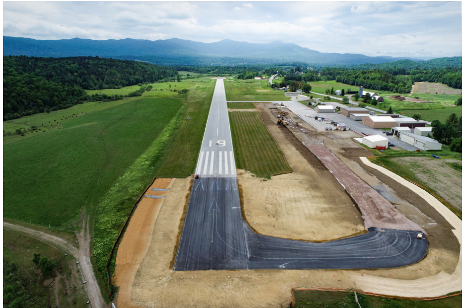
MORRISVILLE-STOWE STATE AIRPORT. Morrisville-Stowe State Airport was busy in the summer of 2021 with improvements to the runway surface area and construction of a new parallel taxiway to create a safer aviation operating environment. These two projects also included earthwork, stormwater drainage, and new electrical infrastructure.
