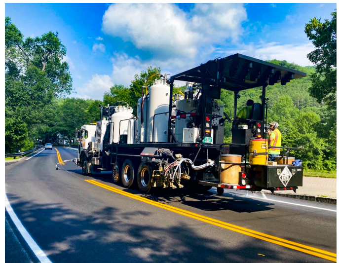
WOODSTOCK. Class 1 paving along US Route 4 and VT Routes 12 and 106 included milling the roadway, paving a new wearing surface, and installing sidewalk ramps, improving pedestrian crossings, and drainage.
