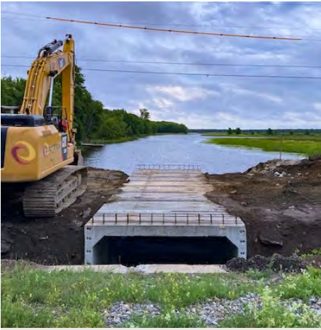
SWANTON. When a washout eroded part of VT Route 78 in late June, AOT crews acted fast and installed a new box culvert in just a few days, enabling this important route through the Champlain Islands to reopen for the Independence Day holiday weekend.
