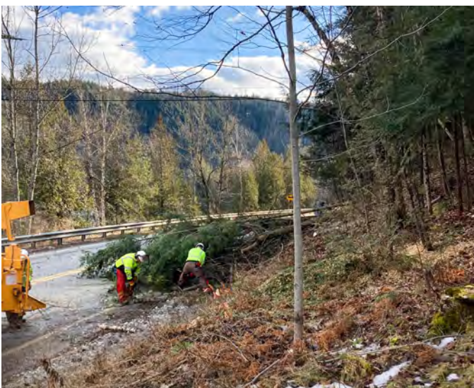
GREENSBORO. Highway maintenance often involves activities off the roadway itself. Our crews stay busy throughout the year cutting back vegetation to help with sight distances and improve safety in the area.
