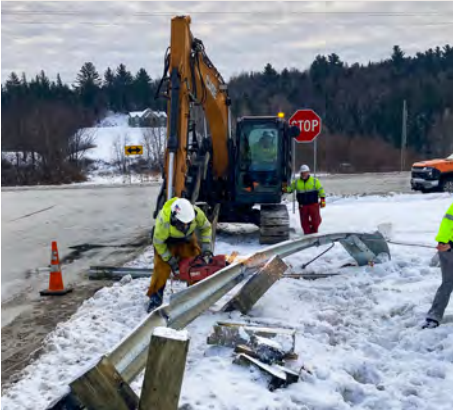
Winter maintenance is about more than just snow plowing. Despite the cold temperatures, VTrans crews spend a good portion of the winter months repairing and replacing damaged guardrails to keep the roadway safe for motorists.
