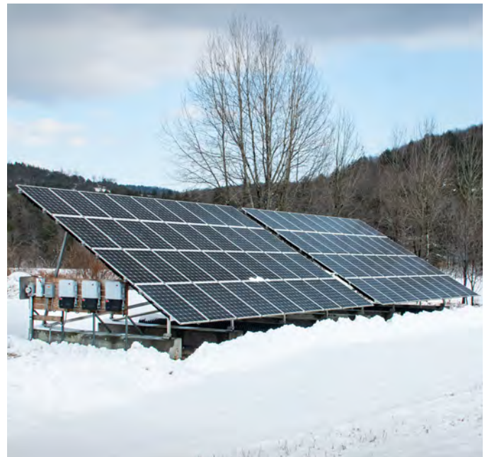
TUNBRIDGE. As the Agency turns to green technologies, one maintenance garage has installed new solar panels and an electric heating system to transition the facilities towards self-sufficiency.
