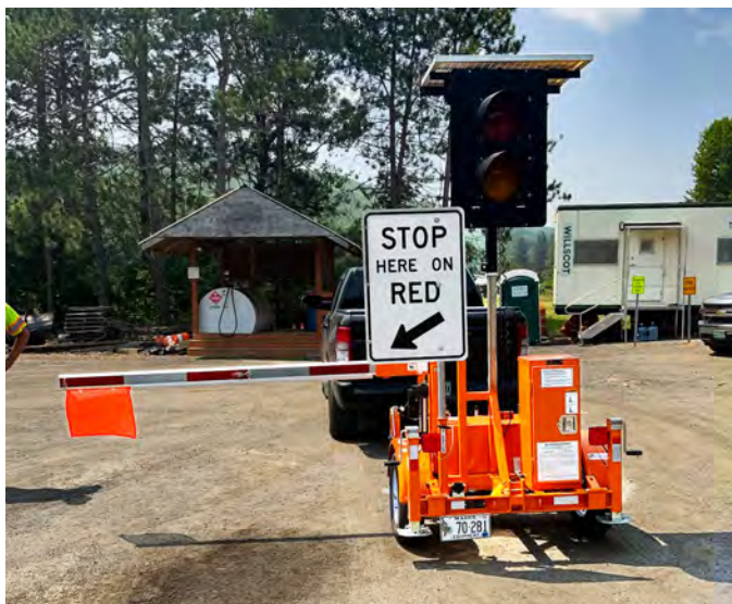
Travelers encountered a new safety technology on the roadway this construction season: Automated Flagger Assistance Devices, or AFADs, are mechanically controlled flagging devices that allow human flaggers to stay out of the roadway while managing the flow of traffic, improving safety for workers and motorists alike.
