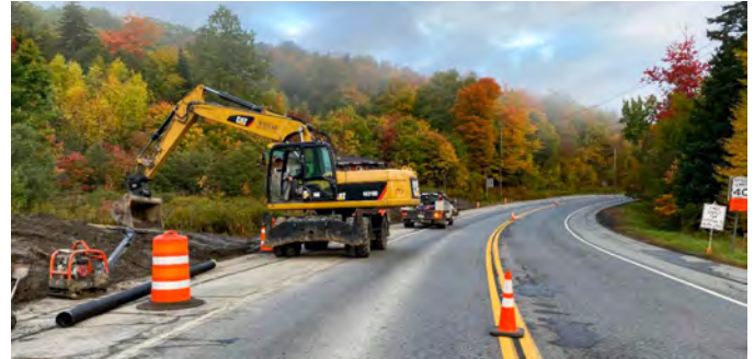
WILMINGTON - BRATTLEBORO. In 2021, a multi-year road reclamation project began along VT Route 9. By 2023, this 12.5 mile stretch of highway will feature new pavement, culverts, guardrail, and other safety improvements.
