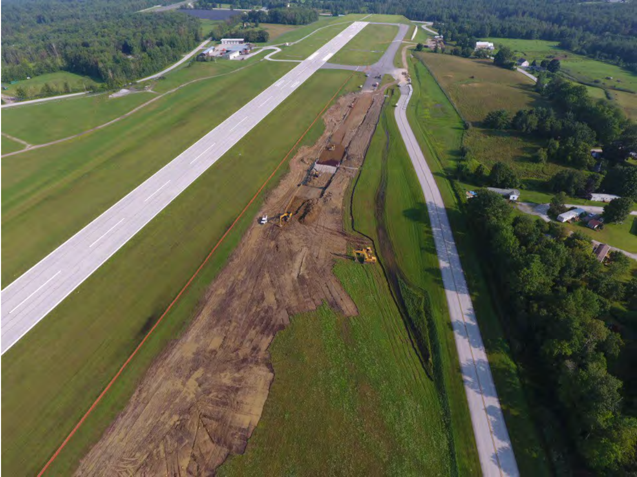
Figure 1. Construction of new Taxiway Alpha "A" at Rutland Southern Vermont Regional Airport
