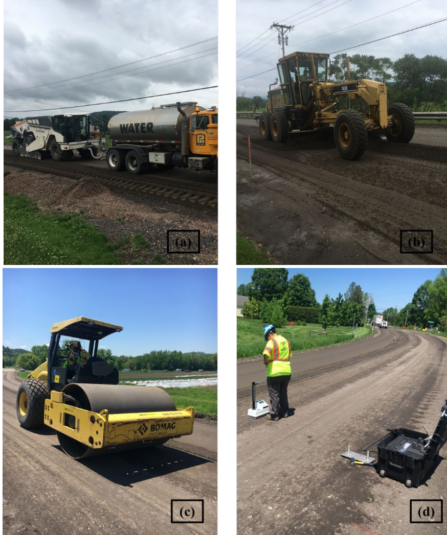
Figure 23. Picture of different road construction equipment (a) Reclaimer, (b) grader, (c) IC roller, and (d) Nuclear Gauge Density
