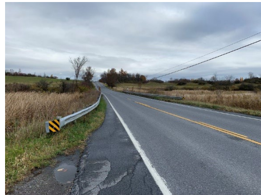
Figure 10. Guardrail with crashworthy end treatment.
