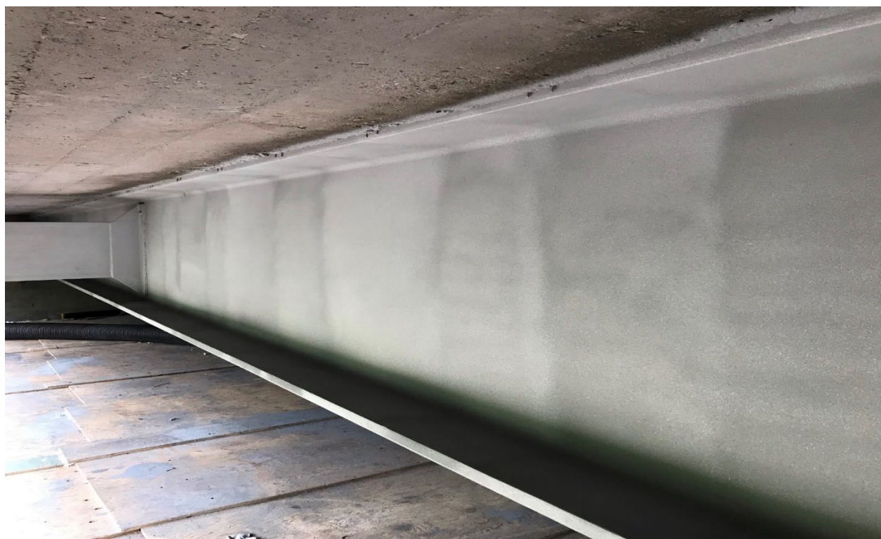
Streaks in the Final Coating
