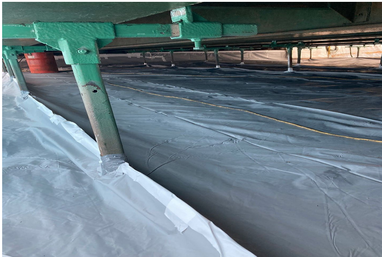
Bottom of Sealed Work Platform
