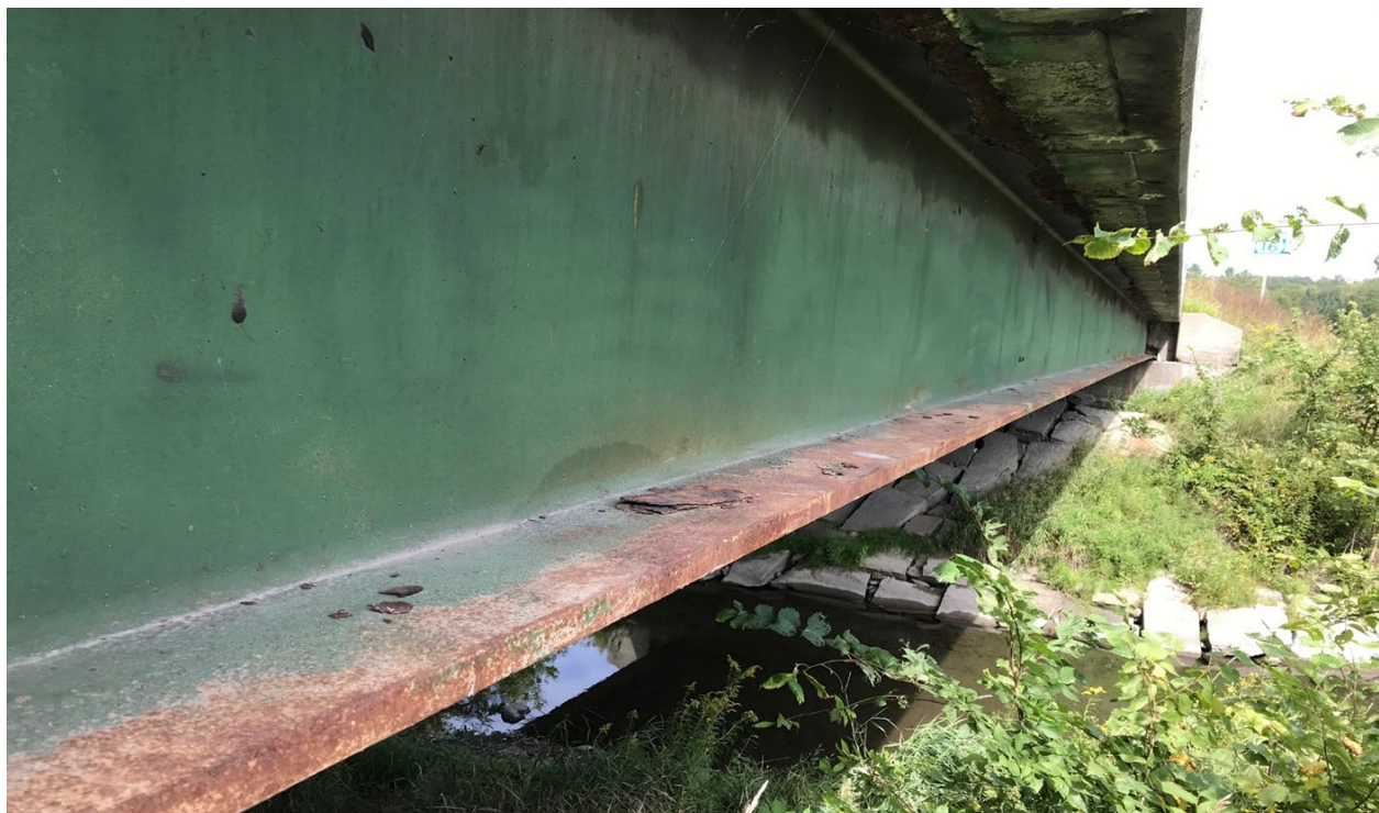
Hardwick VT Br. 1 (Fascia beam paint deterioration)
