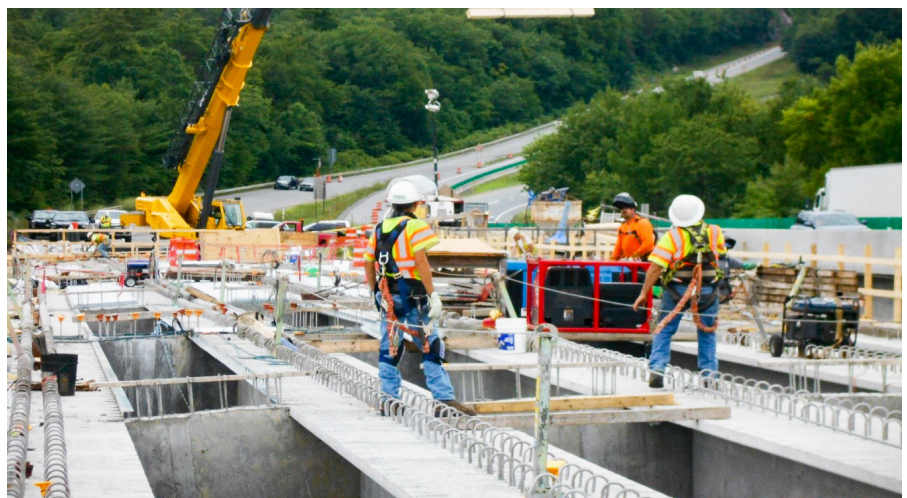
ROCKINGHAM. The multi-year bridge replacement project along I-91 continued in 2020, with the main focus on the building of the new bridge decks. These two new bridges will ultimately feature wider lanes, ensuring safer travel for all.
