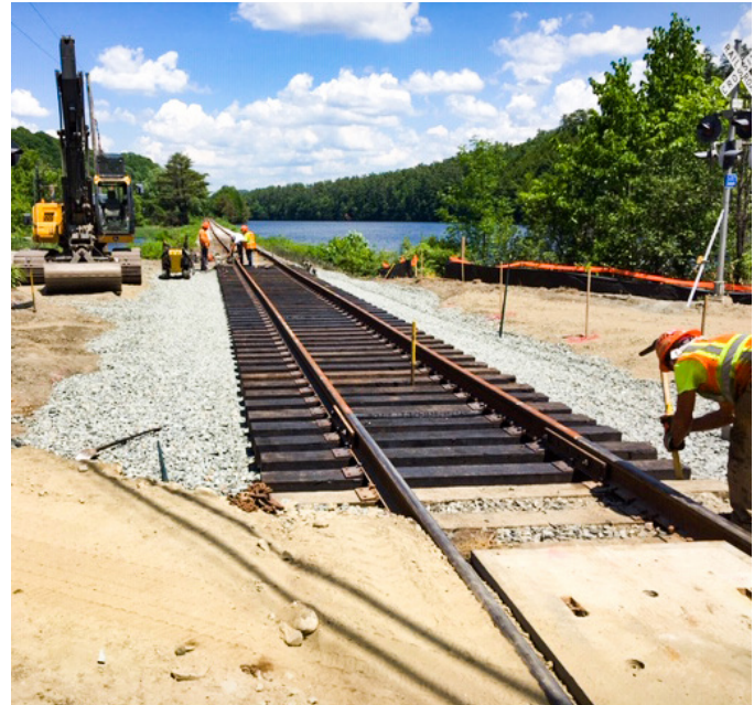
NORWICH. Pictured above is a railroad crossing reconstruction project along River Road in Norwich. The project saw the replacement of concrete surface panels, rail ties, rail ballasts, and the addition of a new active warning signal system with LED lights.
