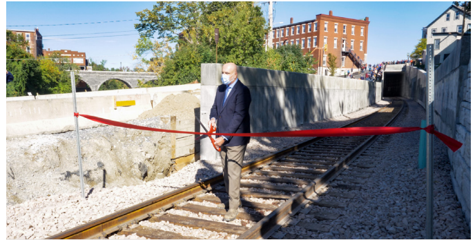
MIDDLEBURY. After many months of excavation and construction, the new rail tunnel in Middlebury officially opened on September 18, 2020. People gathered to witness the first passenger train pass through the tunnel and congregated on Main Street as roads through the downtown were officially reopened.
