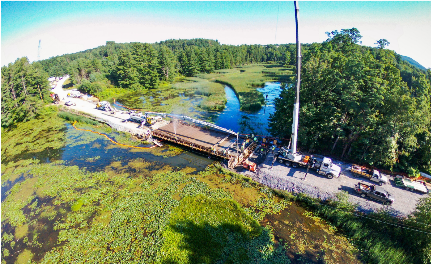
GEORGIA. The replacement of a narrow bridge along VT-104A demonstrated how good planning can rapidly accelerate the construction process. Within the first day of closing the old bridge, the original deck was removed, preparations for the new foundation had begun, and new steel girders arrived on site. Working fast, the project team was able to open the new bridge to traffic within just 37 days.
