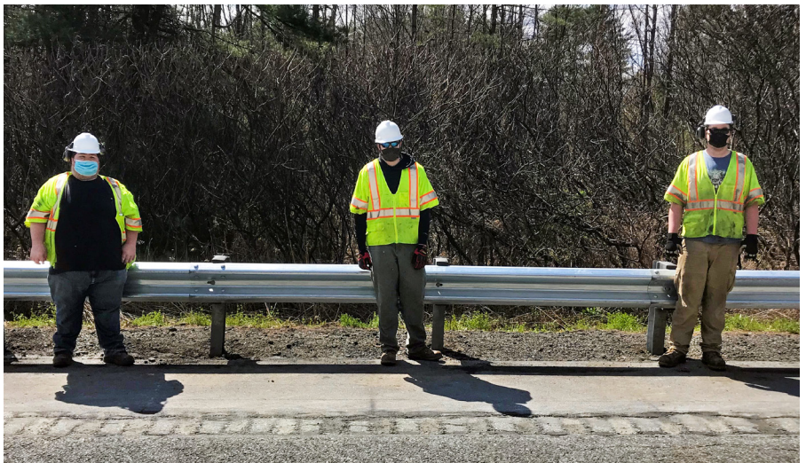
THETFORD. As many students transitioned to online learning, VTrans Intern Maintenance Workers were getting valuable on-the-job experience. Interns from our Thetford garage learned how to repair a damaged guardrail, while social distancing and following safety protocols.
