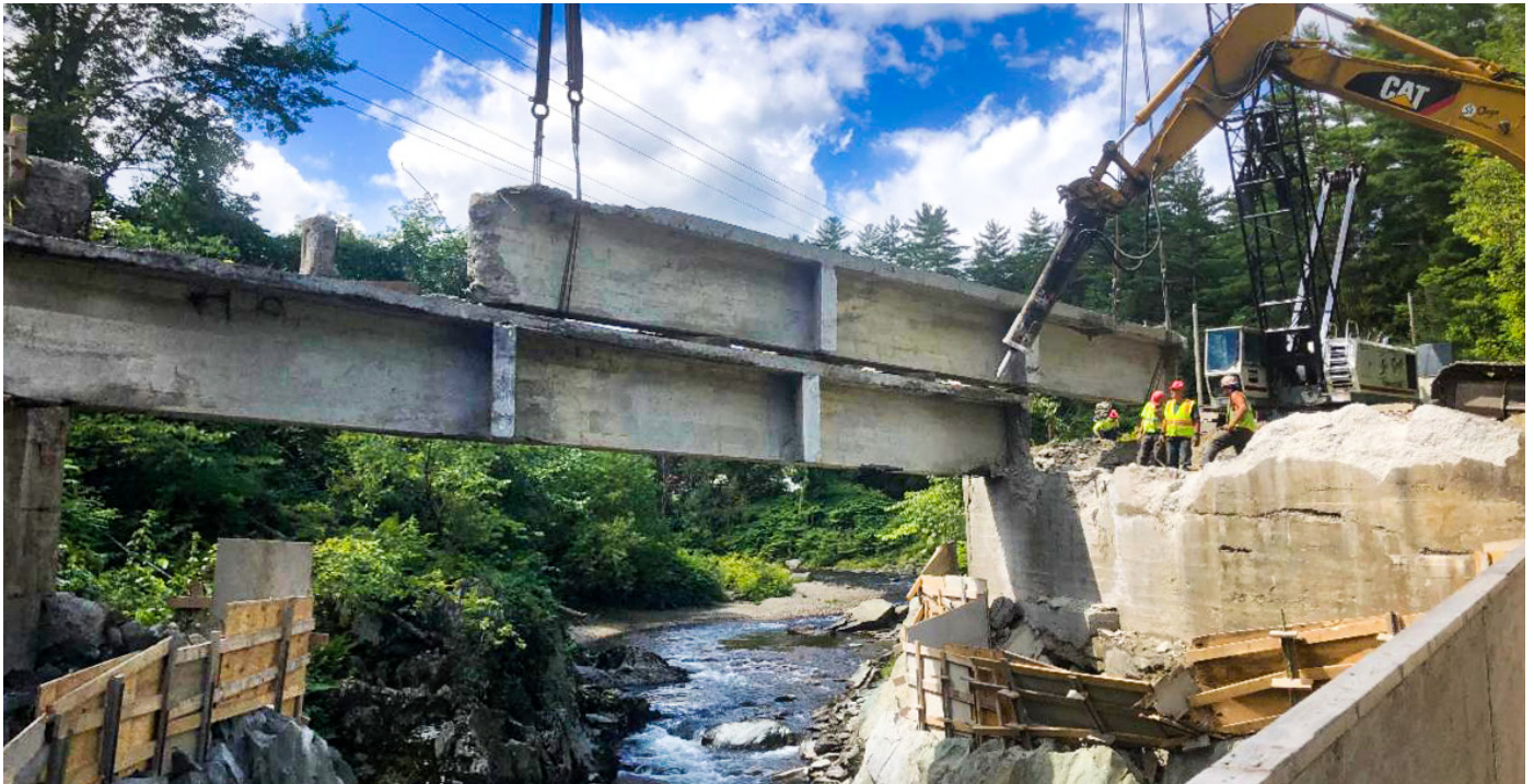
MORETOWN. Built in the 1920s, the original concrete bridge spanning the Mad River along VT-100B was badly in need of replacement. A two-month closure period allowed the old bridge to be demolished quickly, with a new bridge built on a slightly modified alignment. The new structure now spans 100 feet and features wider lanes and shoulders for a safer traveling experience for all.
