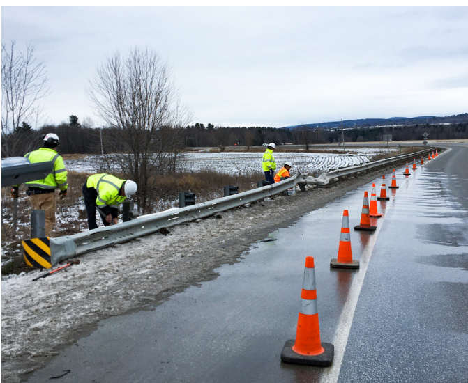
SHELDON. While the cold can be challenging, VTrans crews do as many tasks as winter weather allows. A brief mid-season snow melt enabled crews to take care of badly damaged guardrail along VT-105.
