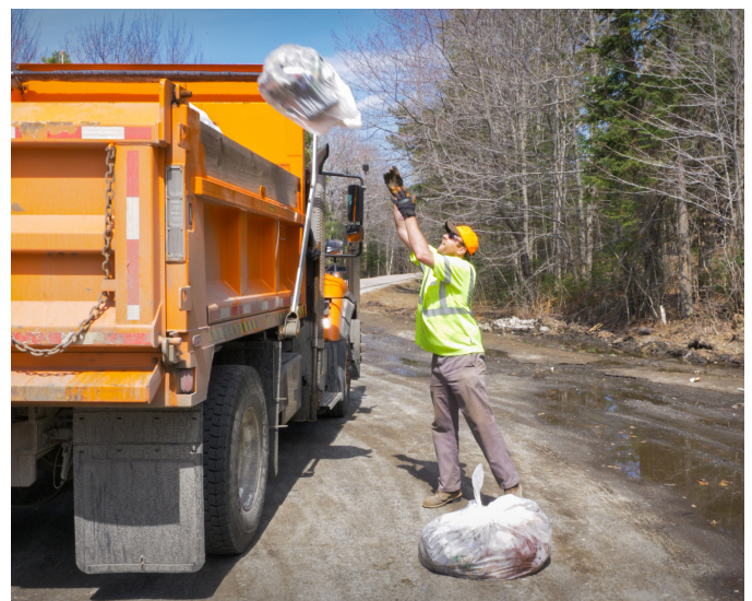
STATEWIDE. While winter keeps our crews busy with snow and ice control, the spring sees VTrans maintenance crews transition from plowing to litter picking, guardrail repair, patching, and more.
