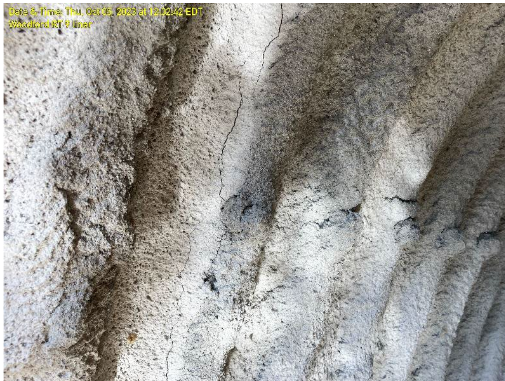
Figure 13. Woodford BR18 Spray On Liner: Minor cracking in barrel (2023)
