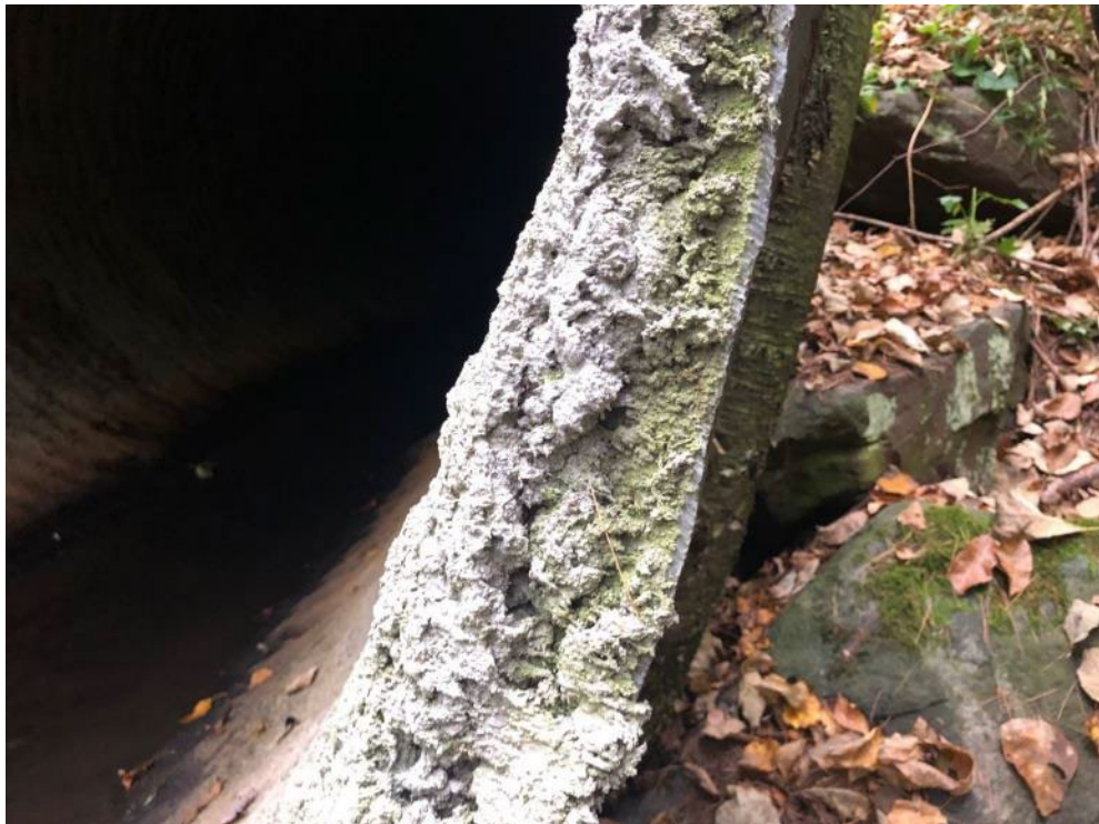
Figure 25. Weathersfield BR15 Spray On Liner: Outlet edge showing signs of algae growth and staining on liner (2023)
