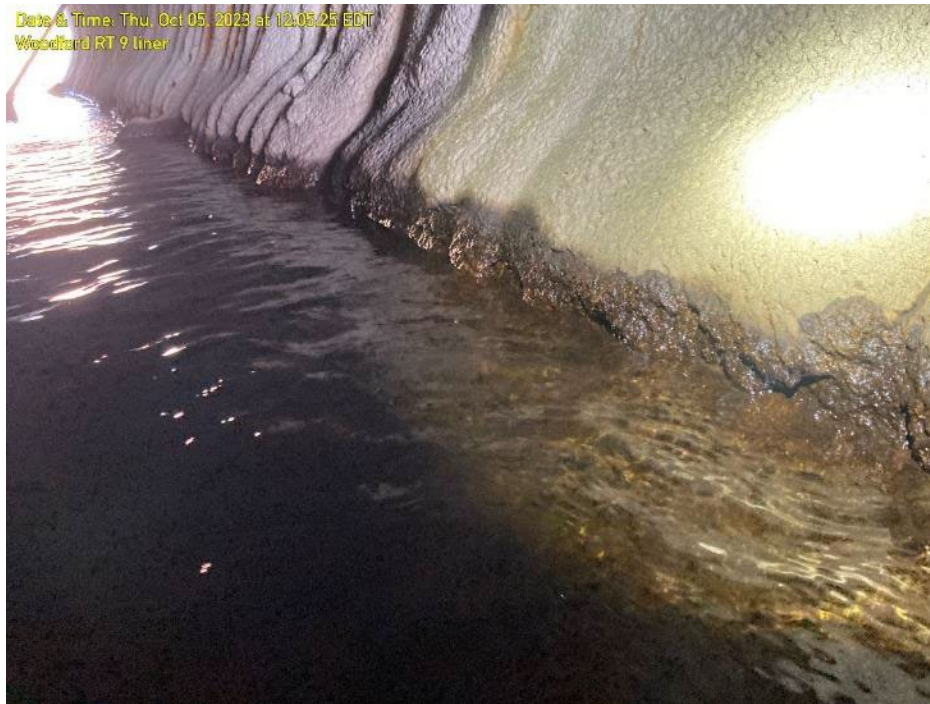
Figure 14. Woodford BR18 Spray On Liner: Invert rust or staining (2023)
