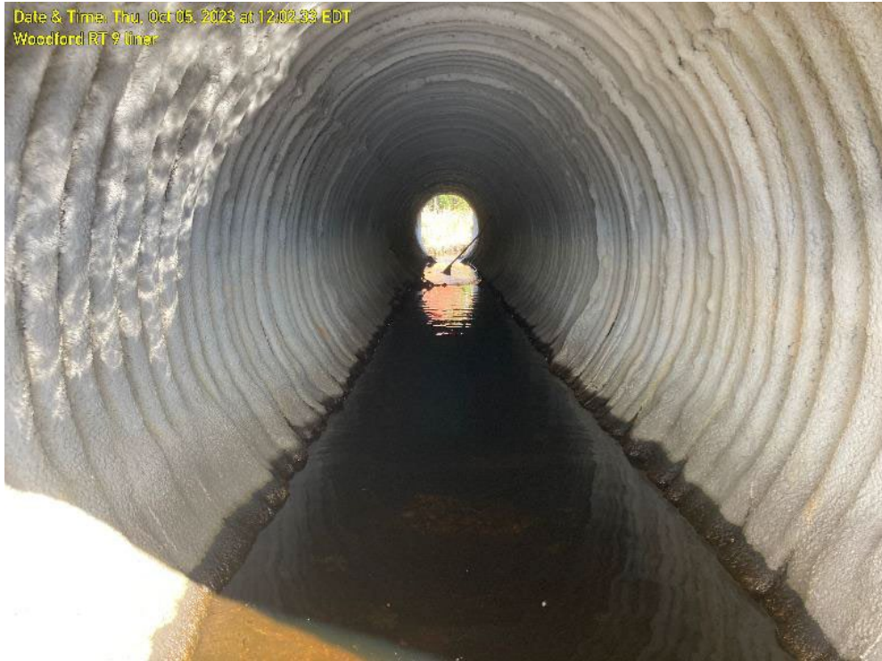
Figure 12. Woodford BR18 Spray On Liner: Barrel condition (2023)
