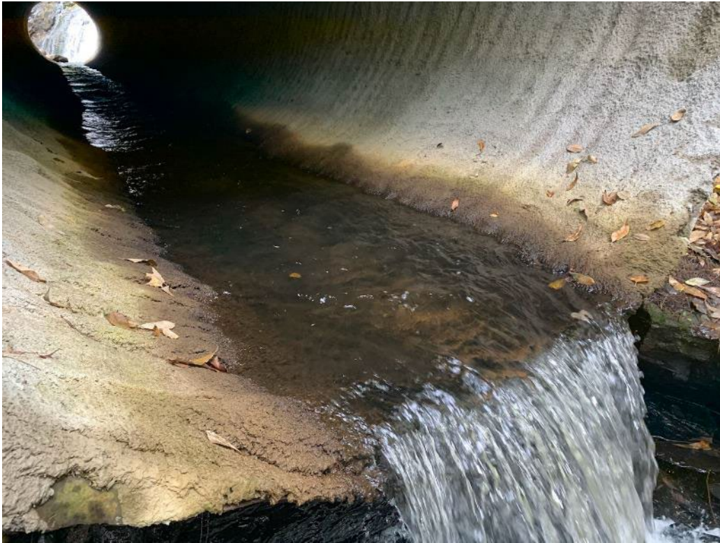
Figure 21. Weathersfield BR15 Spray On Liner: Outlet invert with some minor cracking at pipe edge (2021)
