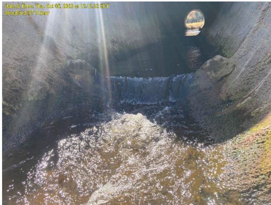
Figure 15. Woodford BR18 Spray On Liner: Fish baffle condition (2023)
