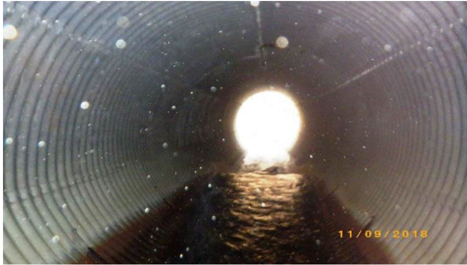
Figure 5. Weathersfield BR15 Barrel Rusting (2018 Inspection Photo)
