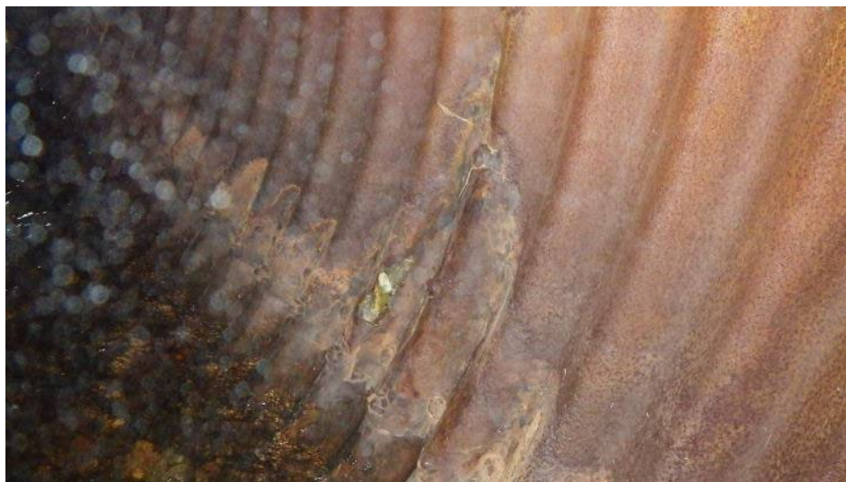
Figure 2. Woodford BR18 Invert Corrosion Damage (2016 Inspection Photo)
