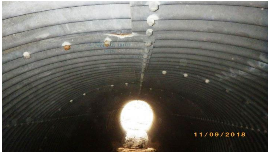
Figure 6. Weathersfield BR15 cracking in plate pipe showing beginning of deformation (2018 Inspection Photo)
