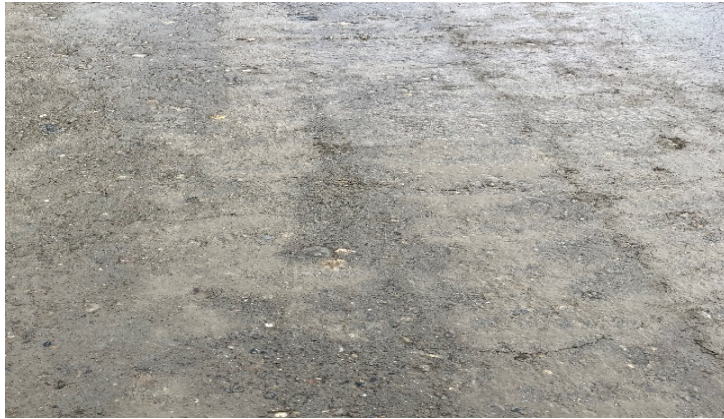
FIGURE 9. MICRO CRACKED FDR SURFACE - PHOTO BY VTRANS
