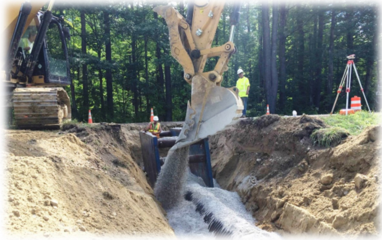
Clarendon Crew - Culvert Failure on Route 7, Wallingford
